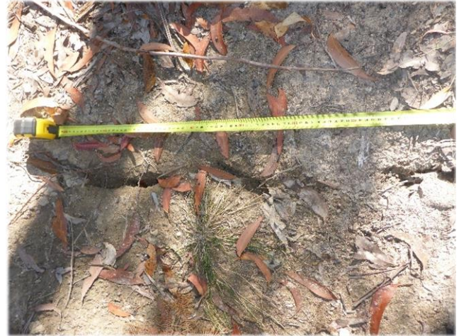
Photo 60: DA3B_LW13_012, largest section of surface cracking. Taken 30th October 2017.
