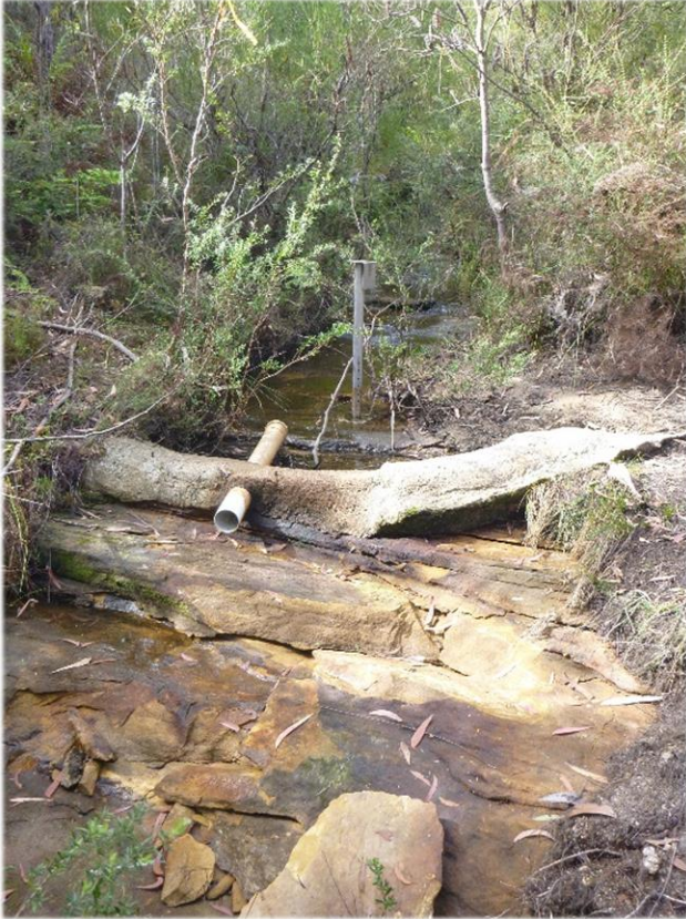
Photo 1: Fracturing downstream from concrete weir, looking upstream. Taken on 19 th April 2017.
