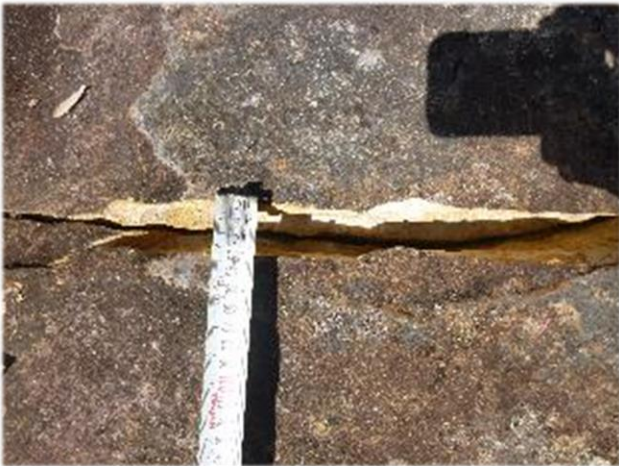
Photo 17: DA3B_LW13_023, closeup of the widest section of fracturing. Taken 29 th March 2018.
