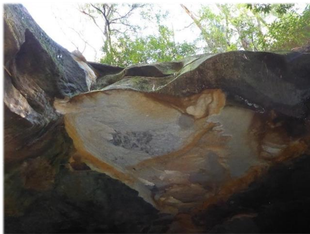
Photo 28: DA3B_LW13_041, looking at the extent of the rockfall. Taken 7 th May 2018.
