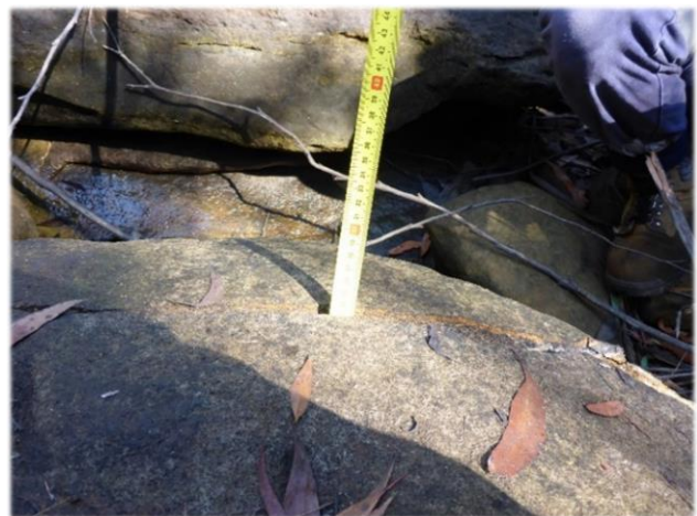
Photo 26: DA3B_LW13_040, looking at the maximum measurable depth of the rock fracturing. Taken 7 th May 2018.
