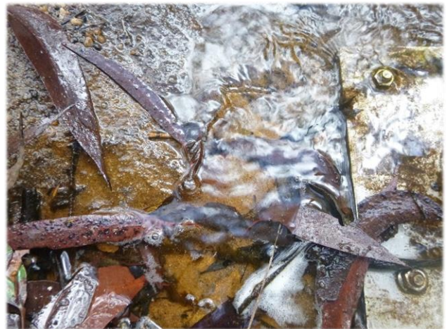
Photo 4: Flow diversion through fracturing in base of pool. Taken on 3 rd May 2017.
