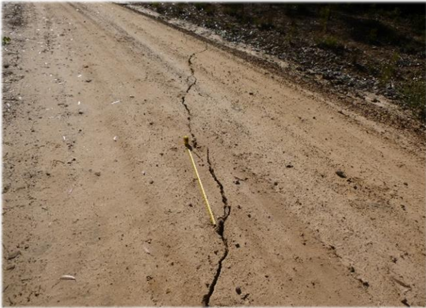
Photo 63: DA3B_LW13_003 , showing the longest continuous section of cracking on FR6A , taken 26 th June 2017.
