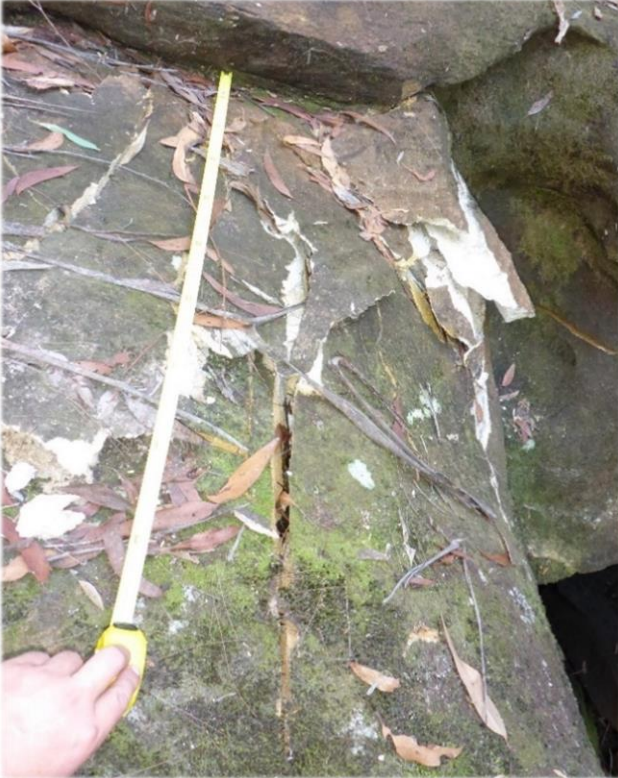
Photo 23: DA3B_LW13_040, looking at a section of rock fracturing and uplift. Taken 7 th May 2018.
