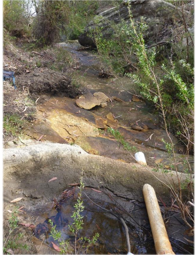
Photo 2: Fracturing downstream from concrete weir, looking downstream. Taken on 19 th April 2017.
