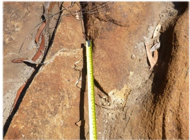
Photo 22: DA3B_LW13_035, looking across stream at the section of plating and uplift. Taken 23 rd April 2018.
