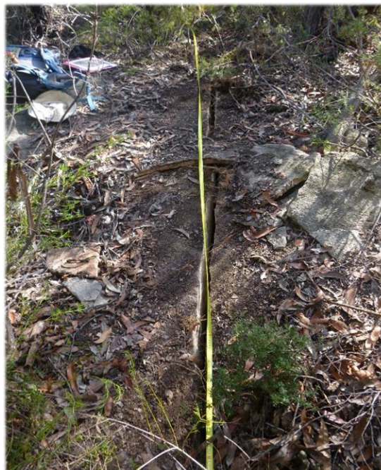
Photo 58: Photo DA3B_LW13_036, looking at the extent of the fracture. Taken 23 rd April 2018.
