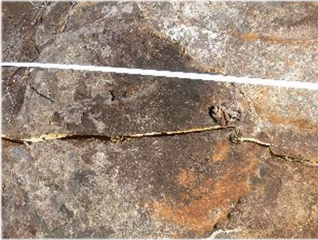
Photo 15: DA3B_LW13_023, widest section of fracturing. Taken 29 th March 2018.
