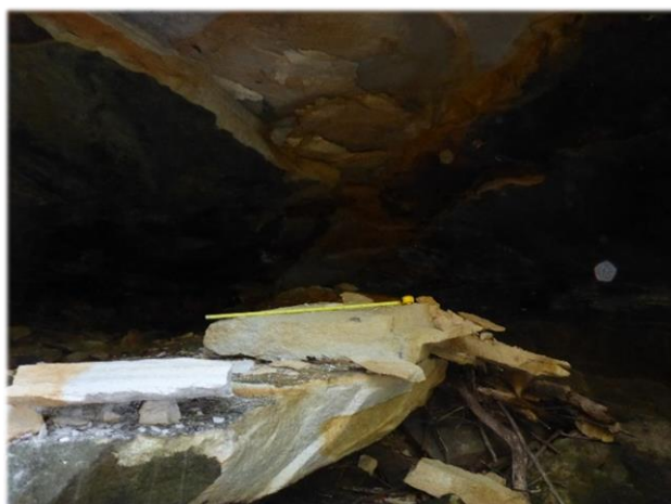
Photo 30: DA3B_LW13_041, looking at the accumulation of rock that resulted from the rockfall. Taken 7 th May 2018.
