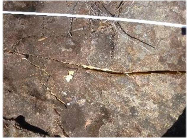
Photo 16: DA3B_LW13_023, widest section of fracturing. Taken 29 th March 2018.
