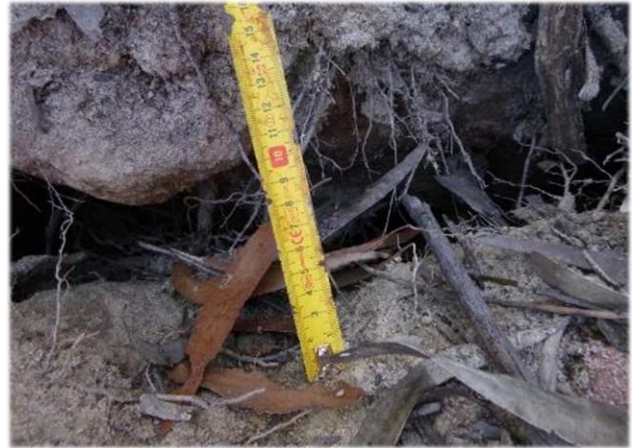
Photo 64: DA3B_LW13_029 , close up of the widest section of cracking. Taken 9 th April 2018.
