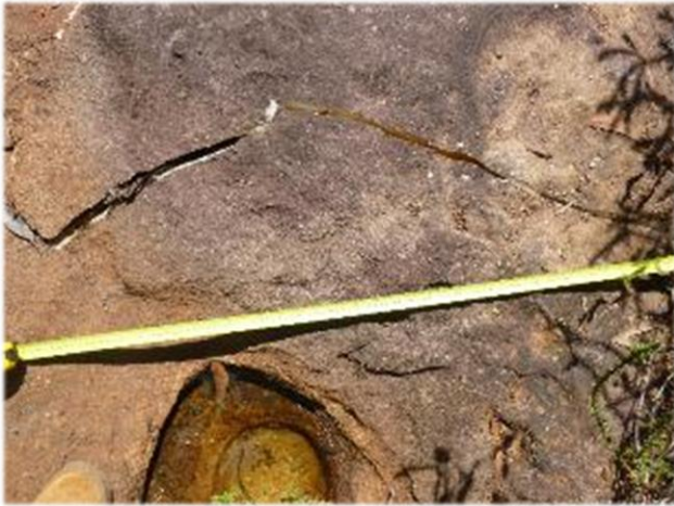
Photo 7: DA3B_LW13_021, looking at the widest section of fracturing. Taken 29 th March 2018.
