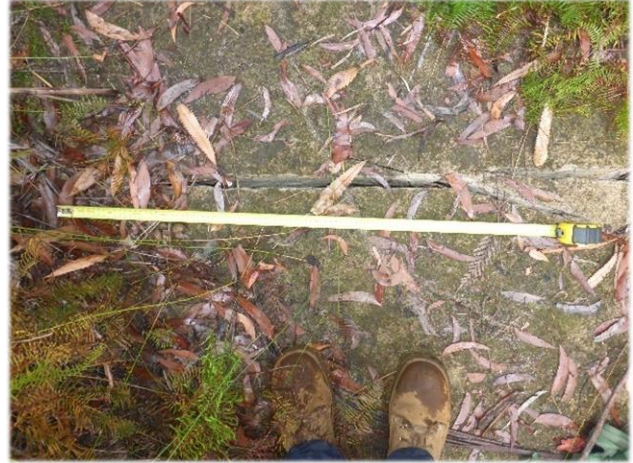
Photo 53: Impact DA3B_LW13_017 , overall extent. Taken on 8/01/2018.
