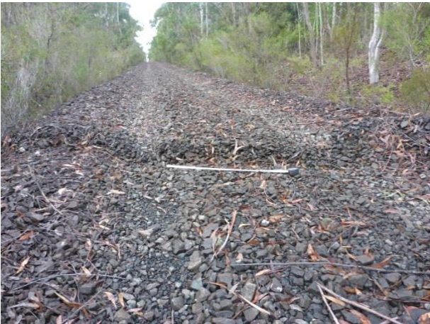
Photo 1: DA3B_LW12_014- Uplift across railway corridor, looking southeast
