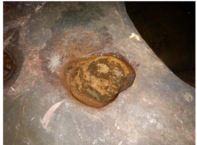
Plate 7 WC21 Pothole C
