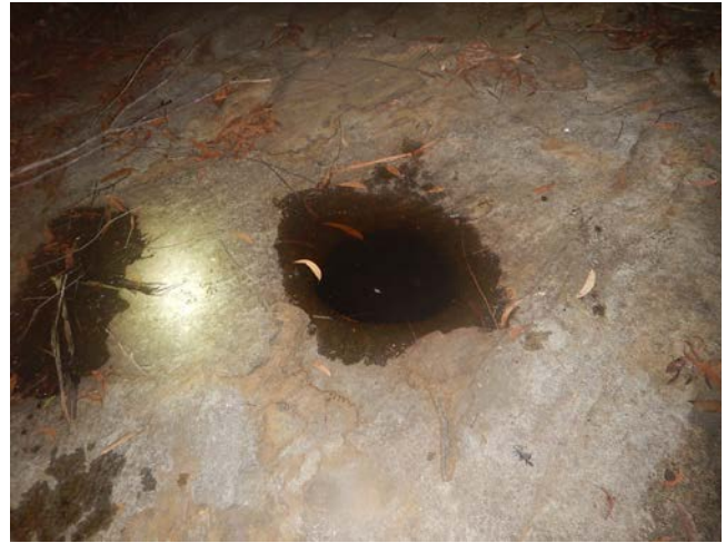
Plate 2 DC13 Pothole B
