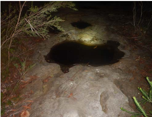
Plate 3 DC13 Pothole C
