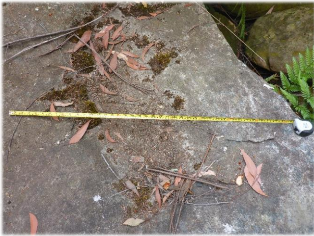
Photo 13: DA3B_LW12_019 - Fracturing to WC21_Rockbar 48 and WC21_Step 48. Taken on 9/11/2016.
