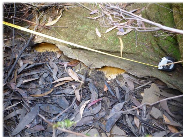
Photo 12: DA3B_LW12_010 - Fracture to channel in LA4b. Taken on 25/05/2016.
