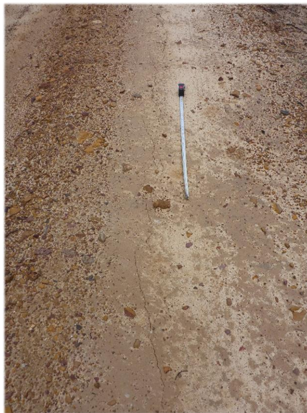
Photo 19: DA3B_LW12_013 – Surface cracking along FR6A. Taken on 27/06/2016.
