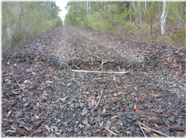
Photo 20: DA3B_LW12_014- Uplift across railway corridor, looking southeast.
