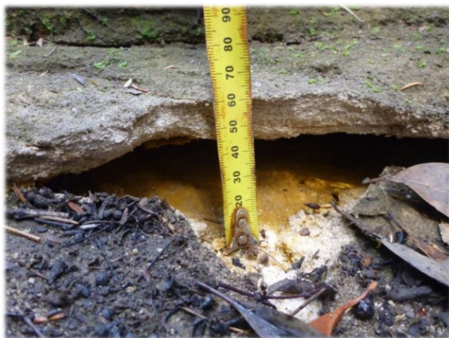
Photo 11: DA3B_LW12_010 - Fracture to channel in LA4b. Taken on 25/05/2016
