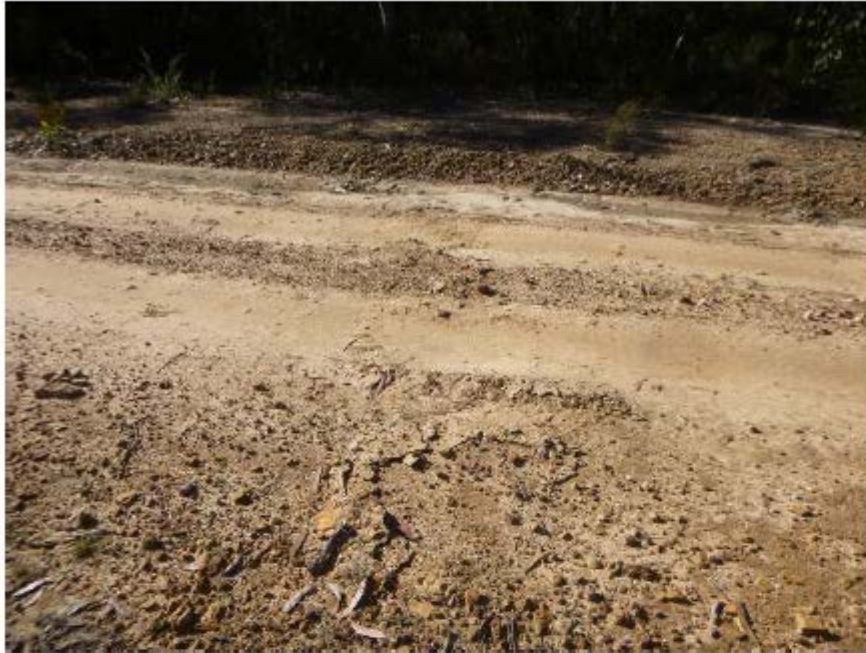
Photo 13: DA3B_LW11_001- Soil crack across Fire Road 6A. Uplift on the southern side of crack is only slightly evident in the photo. Taken on 1/06/2015.
