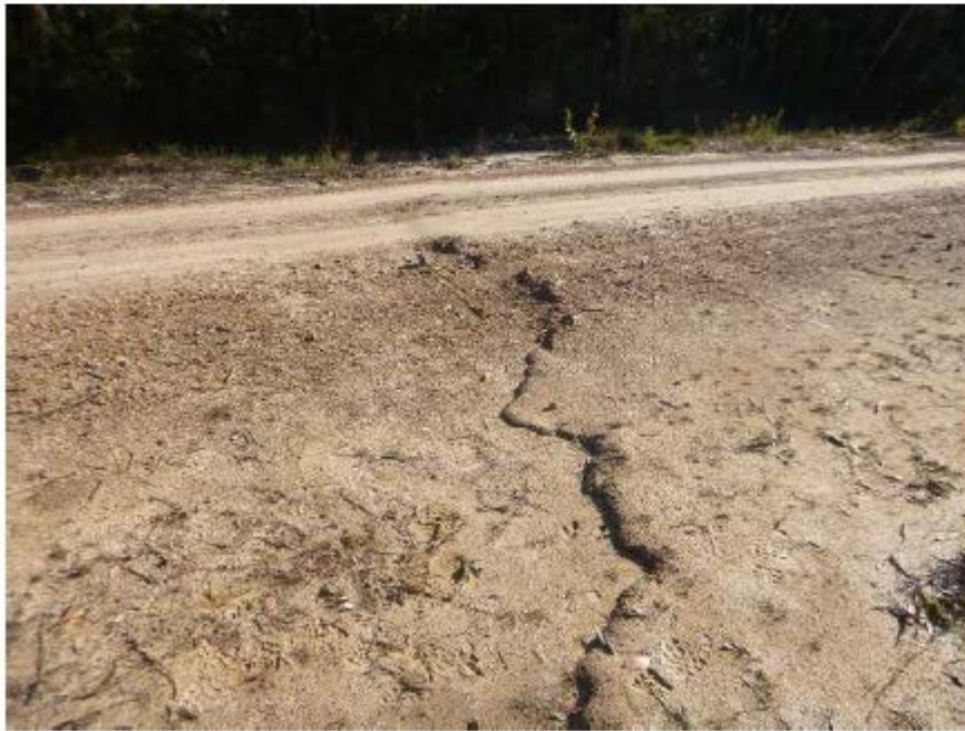
Photo 15: DA3B_LW11_002- Soil crack across Fire Road 6A. Uplift evident on the northern side of crack, more pronounced to the east of Fire Road 6A. Taken on 1/06/2015.
