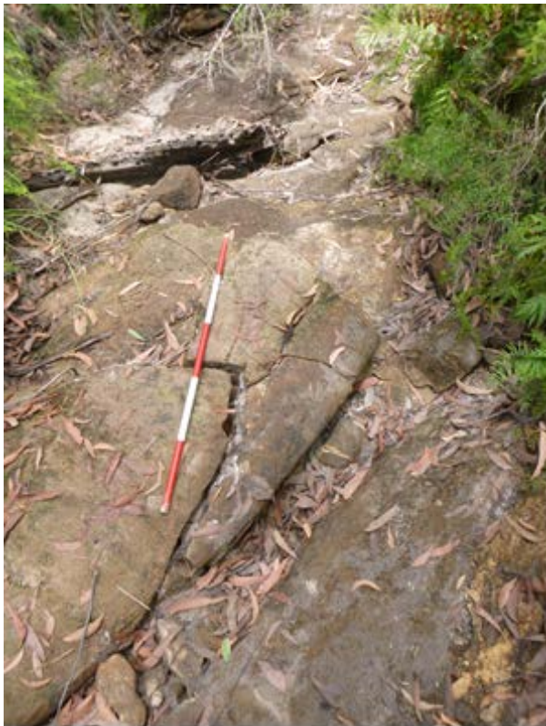
Photo 5: DA3B_LW11_008- Rock fracture, looking upstream along WC21. Taken on 14/01/2016.
