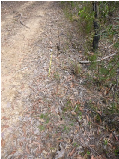
Photo 17: DA3B_LW11_007 Extension - soil crack, looking south along Access Track 6000 (04/02/16).
