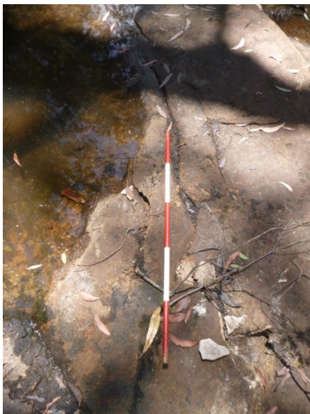
Photo 7: DA3B_LW11_010- Rock fracture, looking upstream along WC21. Taken on 11/02/2016.
