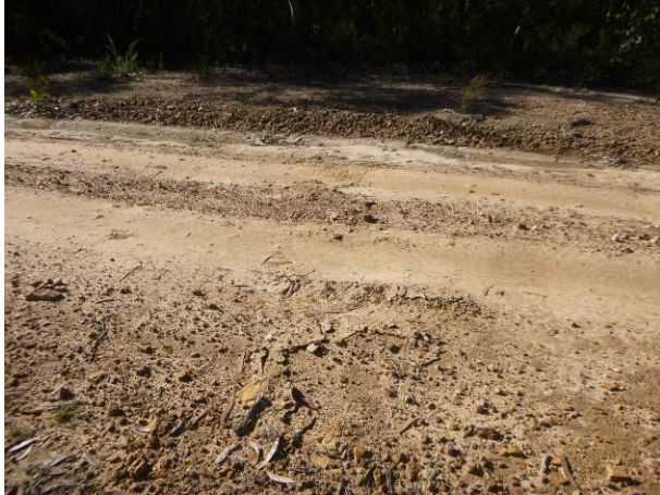
Photo 13: DA3B_LW11_001- Soil crack across Fire Road 6A. Uplift on the southern side of crack is only slightly evident in the photo. Taken on 1/06/2015.
