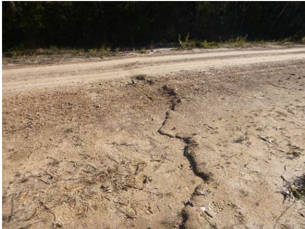
Photo 15: DA3B_LW11_002- Soil crack across Fire Road 6A. Uplift evident on the northern side of crack, more pronounced to the east of Fire Road 6A. Taken on 1/06/2015.
