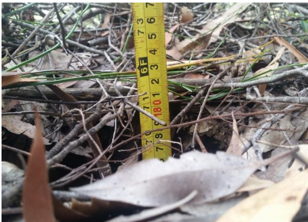
Photo 14: Impact DA3B_LW10_024. Depth of crack. Taken on 18/02/2015
