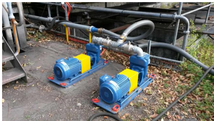
Figure 9: Newly installed GWTP pumps
