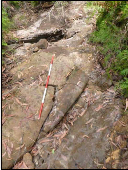
Photo 43: Impact LW11_008- Rock fracturing to upstream from WC21_Pool 30, looking upstream. Taken on 14 January 2016.
