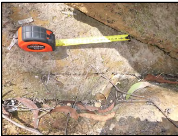
Photo 111: Impact DA3B_LW9_014- fracturing to rock shelf adjacent to WC21_Pool 16. Taken on 10 December 2013.
