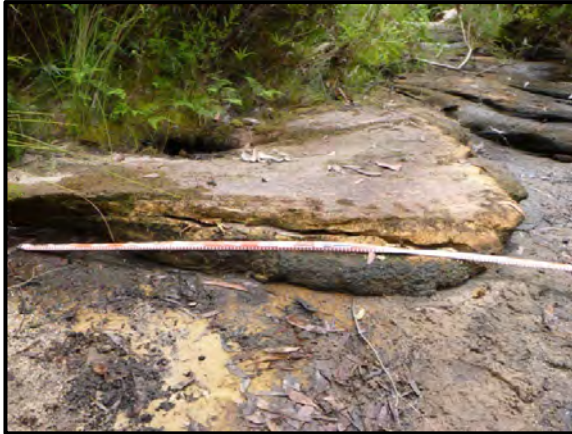
Photo 65: Impact LW10_011- fracturing with dislodged fragment on Rockbar 24, looking downstream. Taken 25 November 2014.
