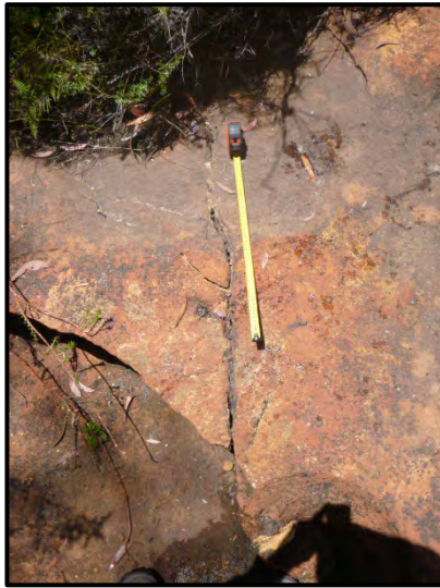
Photo 105: Impact LW9_016, dilation of joint looking across stream. Taken on 17 December 2013.
