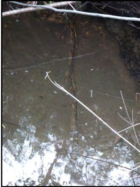
Photo 62: Impact LW10_010- dilation of joint on base of pool, looking downstream. Taken on 25 November 2014.
