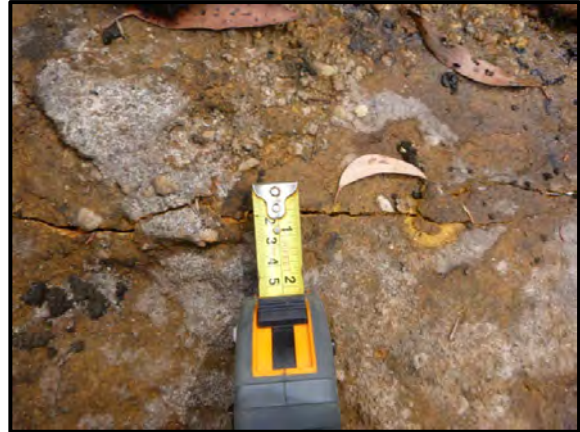
Photo 83: Impact DA3B_LW10_014- Fracture to base of WC21_Pool 23. Photo taken on 4 December 2014.
