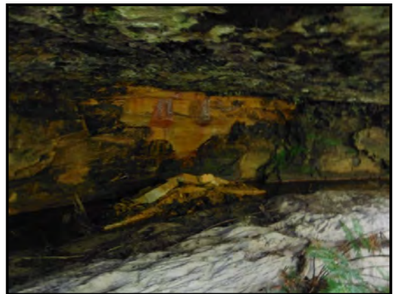
Photo 127: Impact LW9_028, small rockfall to overhang adjacent to Pool 10. Taken on 17 March 2014.
