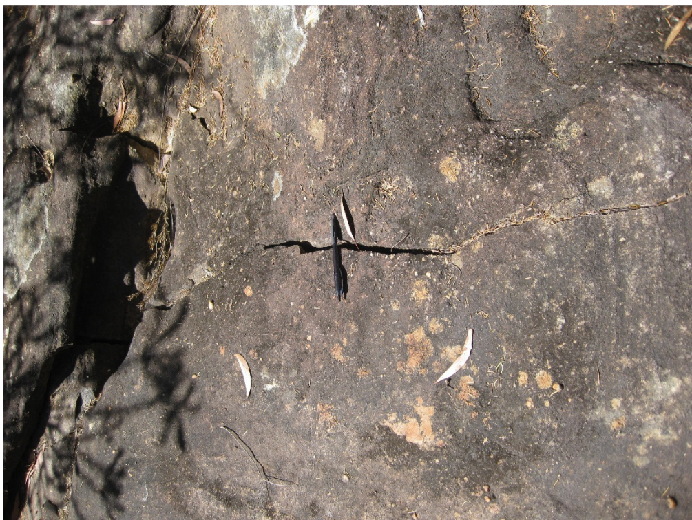
Photo 2 - Cracked Rock Bar along 2nd Order Creek No. WC21, Area 3B (>2 years since mining of LW 10)
