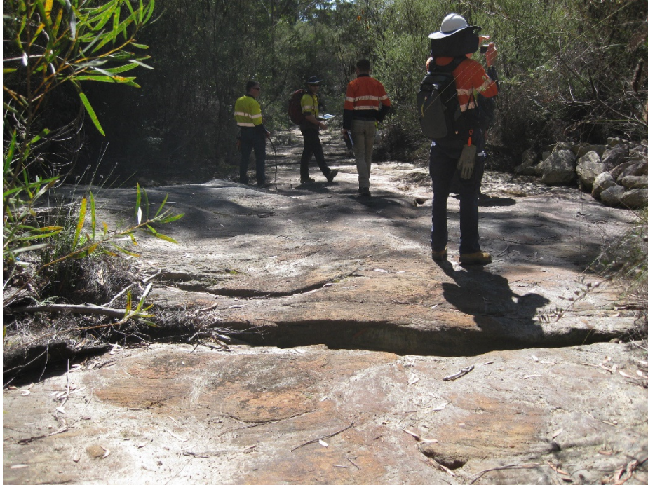
Photo 1 - Inspection of Rock Bar Cracking along 2nd Order Creek No. WC21, Area 3B (>2 years since mining of LW10)
