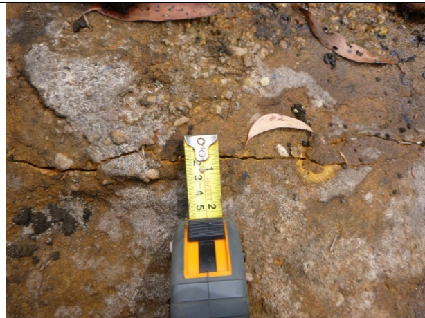
Photo 32: Impact DA3B_LW10_014-Fracture to base of WC21_Pool 23. Photo taken on 4/12/2014.
