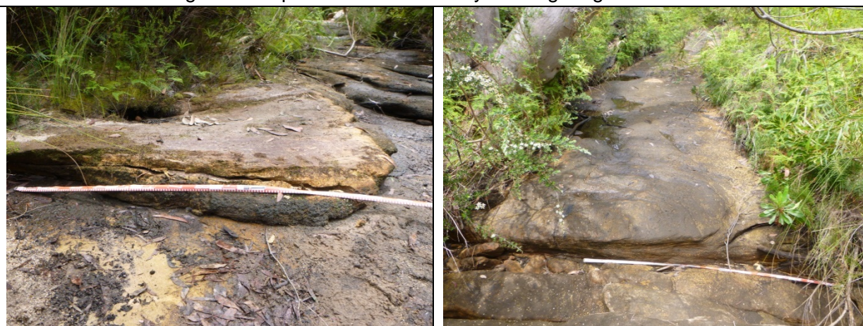
Photo 14: Impact LW10_011- fracturing with dislodged fragment on Rockbar 24, looking downstream. Taken on 25/11/2014.
