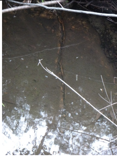
Photo 11: Impact LW10_010- dilation of joint on base of pool, looking downstream. Taken on 25/11/2014.
