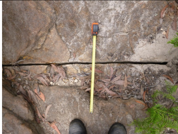
Photo 48: Impact LW9_021- Rock fracturing to Rockbar 18. Taken on 2/01/2014.
