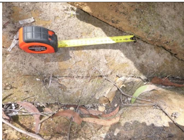
Photo 60: Impact DA3B_LW9_014- fracturing to rock shelf adjacent to WC21_Pool 16. Taken on 10/12/2013.
