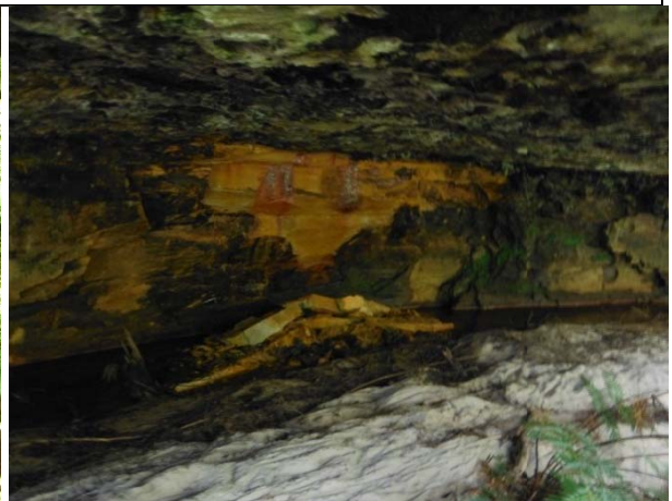
Photo 76: Impact LW9_028, small rockfall to overhang adjacent to Pool 10. Taken on 17/03/2014.
