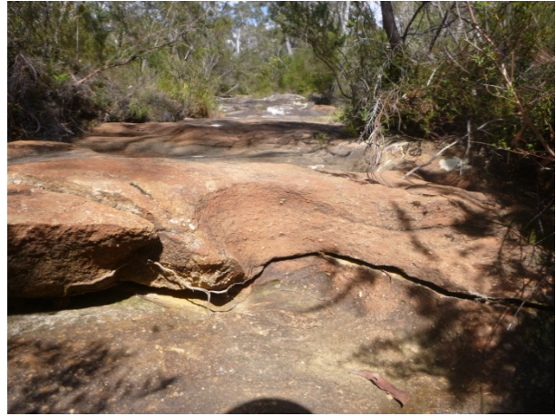
Photo 55: Rockbar 17, looking upstream at fracturing. Taken on 10/09/2015.
