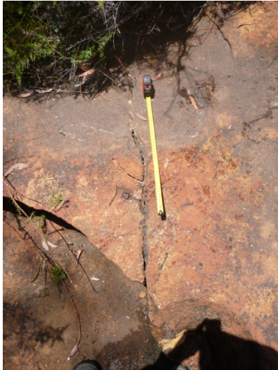
Photo 54: Impact LW9_016, dilation of joint looking across stream. Taken on 17/12/2013.
