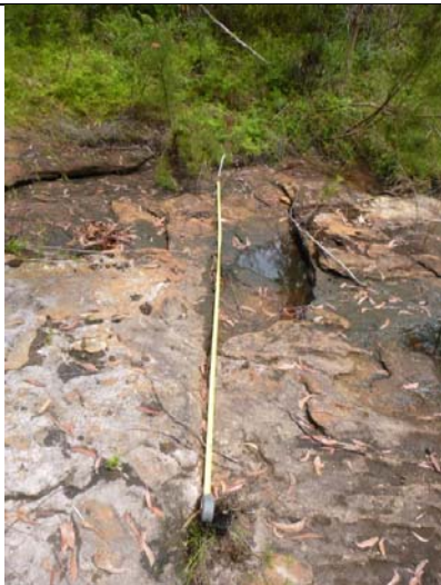
Photo 45: Impact LW10_016- Rock fracture extending across rockbar and through joint, looking across stream. Taken on 04/12/2014.
