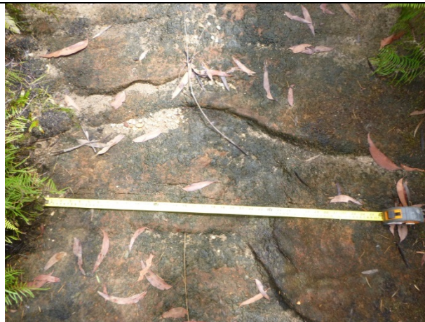
Photo 33: Impact DA3B_LW10_015-Fracturing downstream from WC21_Pool 23, looking upstream. Photo taken on 4/12/2014.
