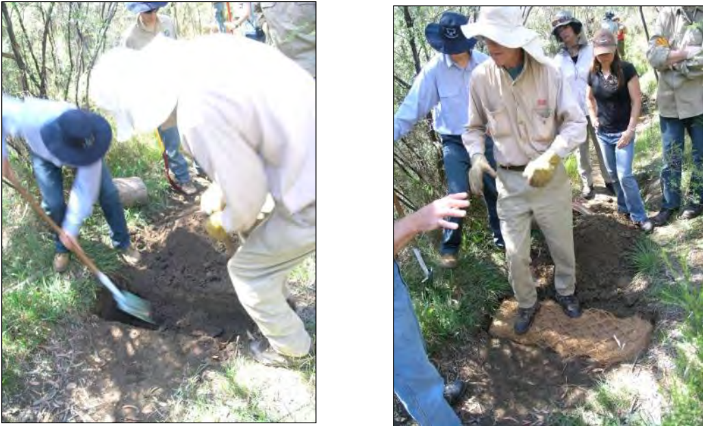
Figure 5-4 Trenching and Positioning of the First Layer of Coir Logs and Construction of a Small Dam in a Channel
