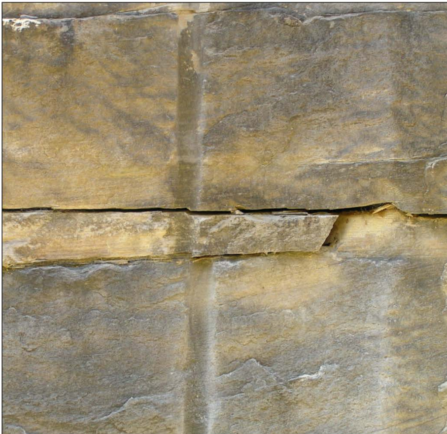
Figure 4: Examples of mining induced shear movements causing offsets and associated vertical fracturing.
