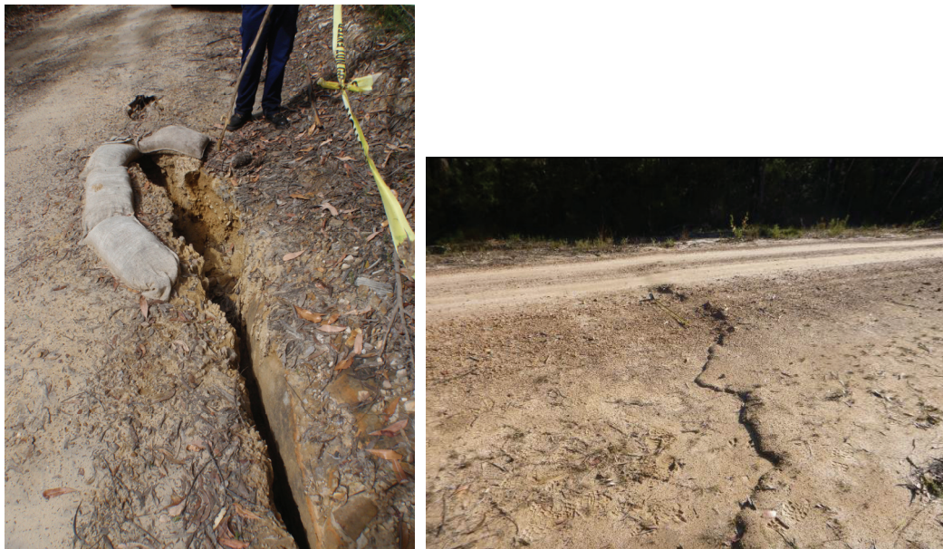
Fig. 6.2 Impacts along the unsealed roads and tracks above LW6 in Area 3A (left side) and above LW11 in Area 3B (right side) (Source: IC)
