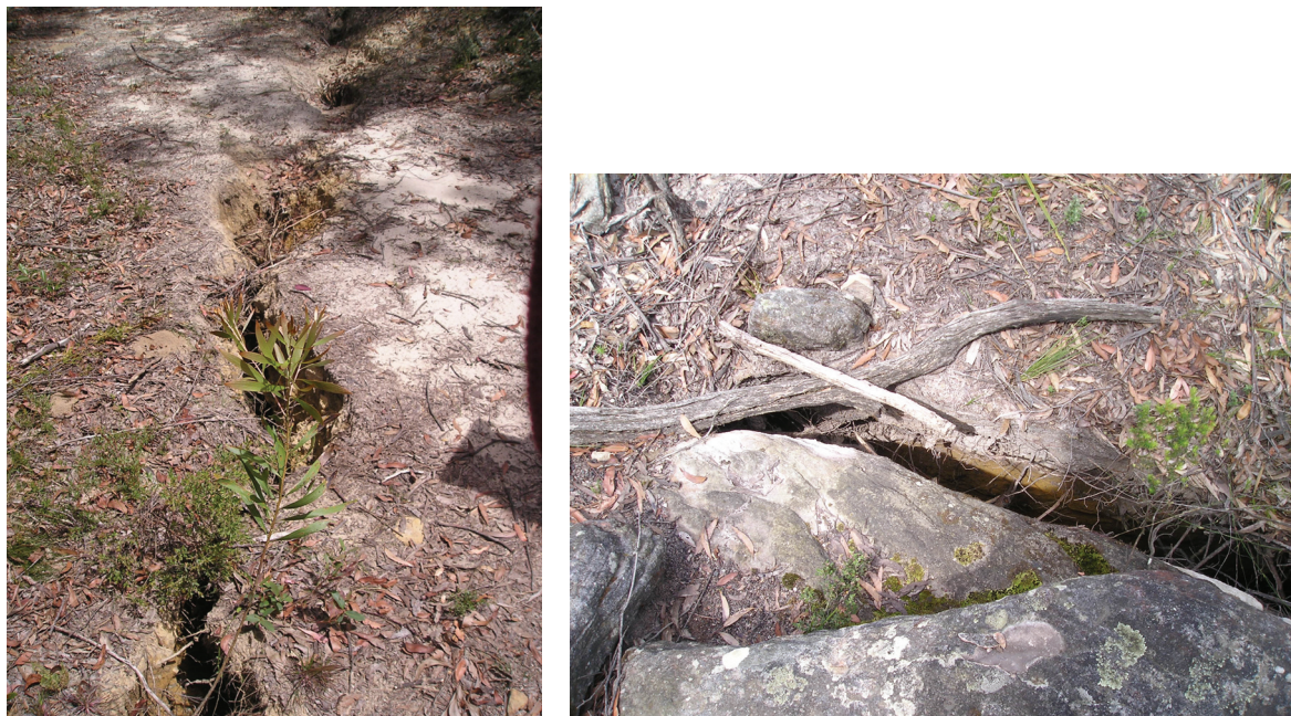
Fig. 5.13 Surface tension cracking due to downslope movements at Dendrobium Mine
