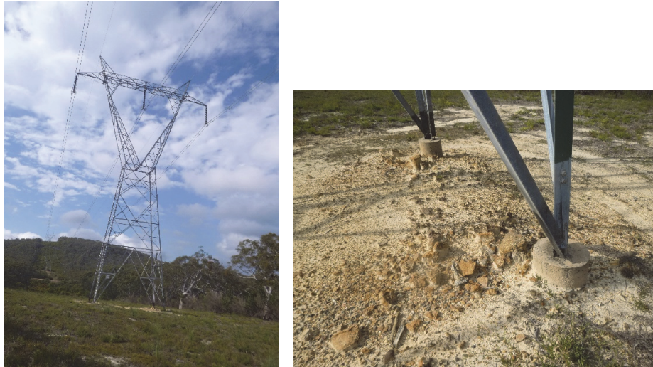
Fig. 6.3 330 kV transmission tower
