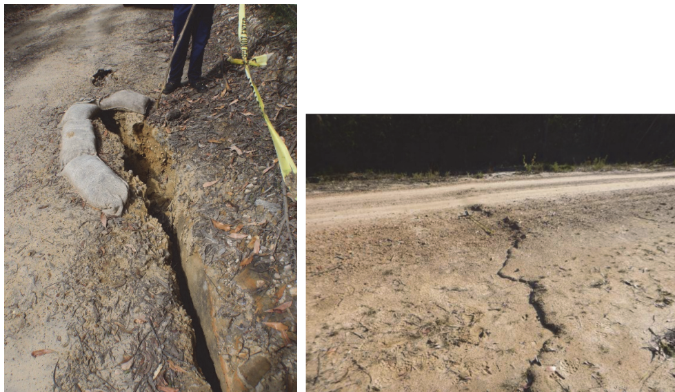
Fig. 6.2 Impacts along the unsealed roads and tracks above LW6 in Area 3A (left side) and above LW11 in Area 3B (right side) (Source: IMC)
