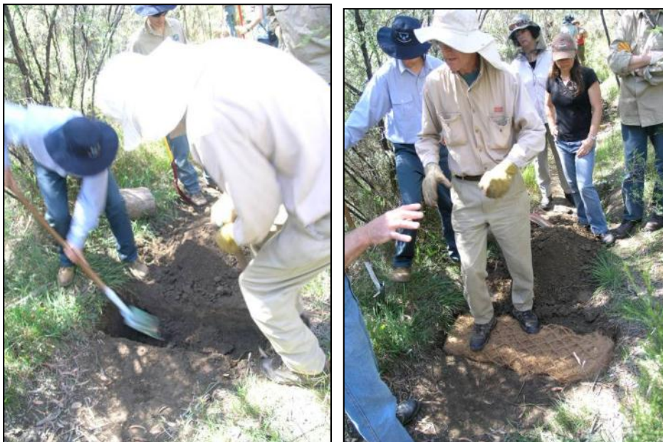
Figure 5-4 Trenching and Positioning of the First Layer of Coir Logs and Construction of a Small Dam in a Channel
