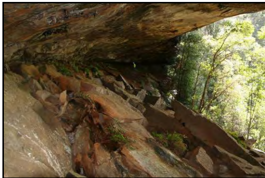
Plate 115: Roof fall at DM23
