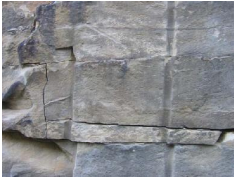
Fig. 5.10 Fracturing in the Rock Cuttings above the Previously Extracted Elouera Longwalls
