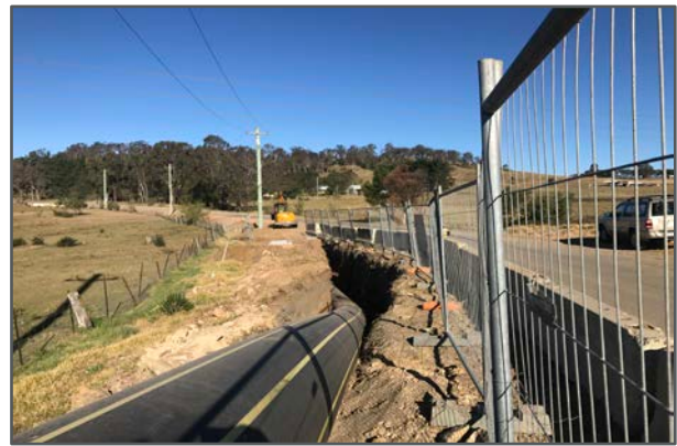
Figure 4: Buried gas pipeline along Brooks Point Road during the construction phase of the project.
