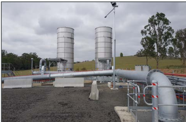
Figure 3: Gas flaring units constructed at the Appin East GDP.
