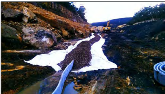
Figure 1: Extending the emplacement underdrainage network as Stage 3 coalwash emplacement progresses down the valley.
