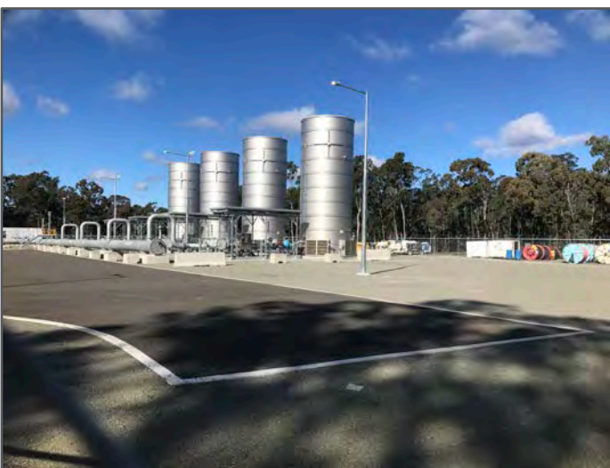
Figure 3: Upgraded gas drainage plant at Appin West
