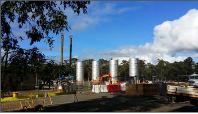
Figure 3 Upgraded gas drainage plant at Appin West.
