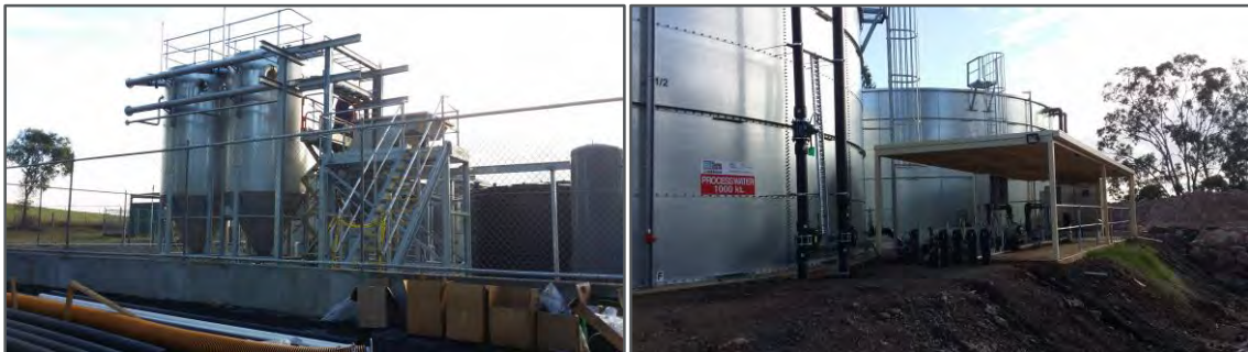
Figure 2: Pre-treatment Plant and storage tanks.
