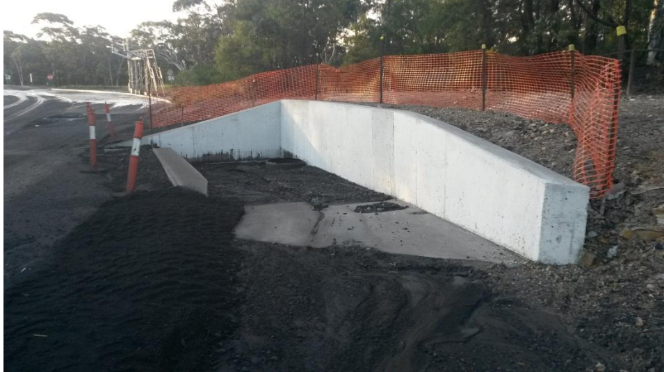
Figure 3: New sediment sump near completion. Under-road drainage pipe (as per table above) exits sump on left of frame.
