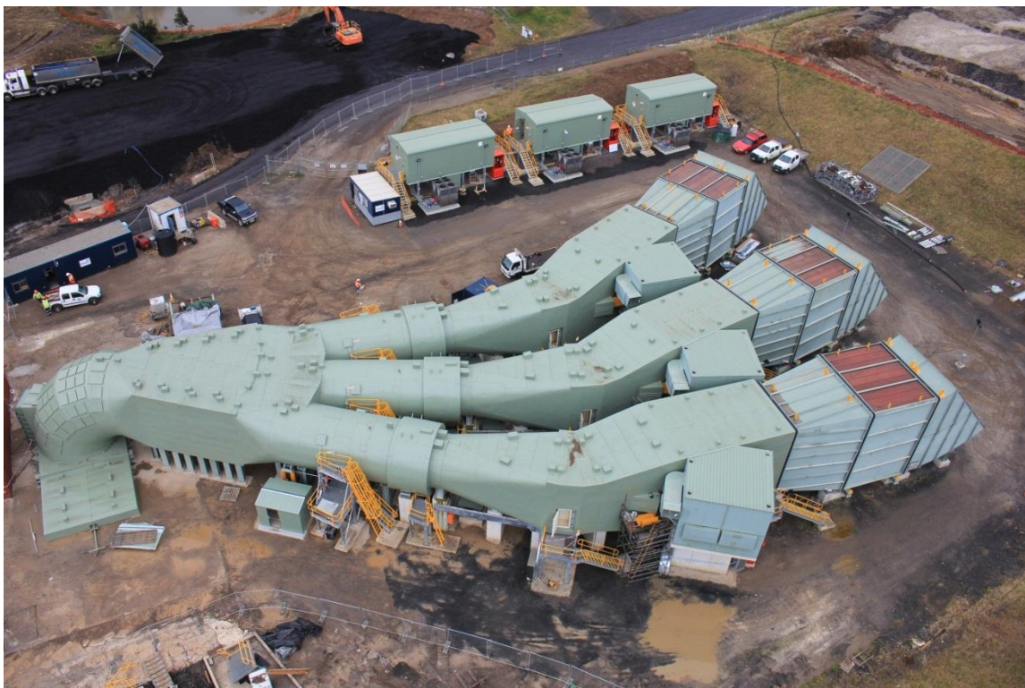
Figure 1: An elevated view of the VS#6 precinct during commissioning. Three fan housings (centre) and ducting connecting to the vent shaft (left).
