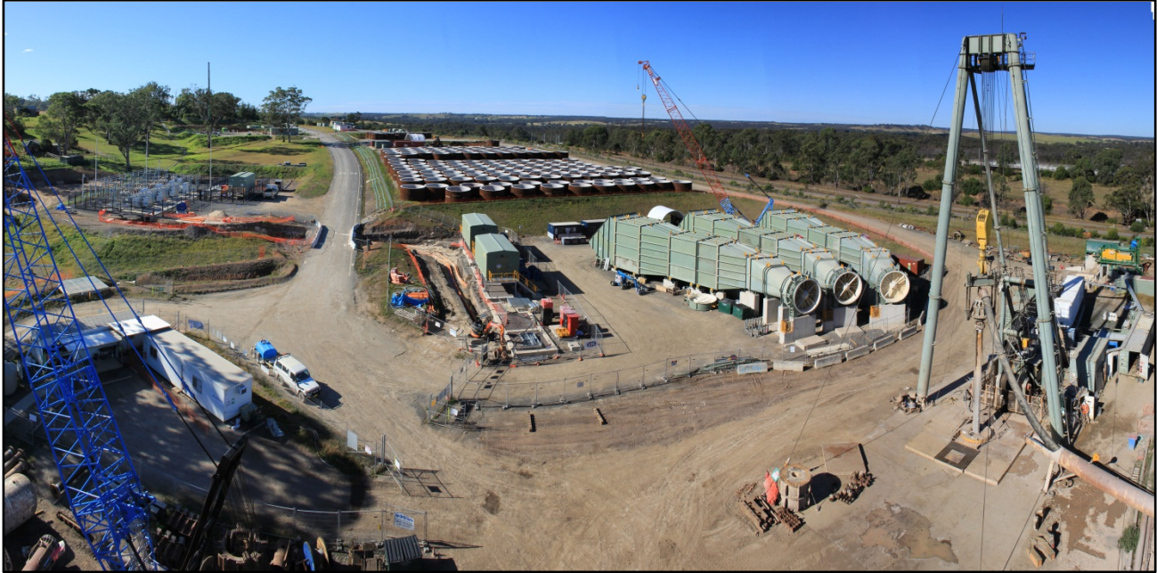
Figure 1: An elevated view of the VS#6 precinct showing the shaft drilling activities (foreground on right), fan and ducting construction (green structure behind drill rig), shaft liners (background on right), and electrical substation (centre on left).
