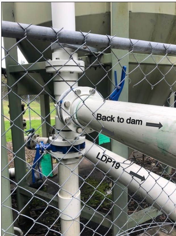
Plate 1: Recirculating valve after Dynasand filter
