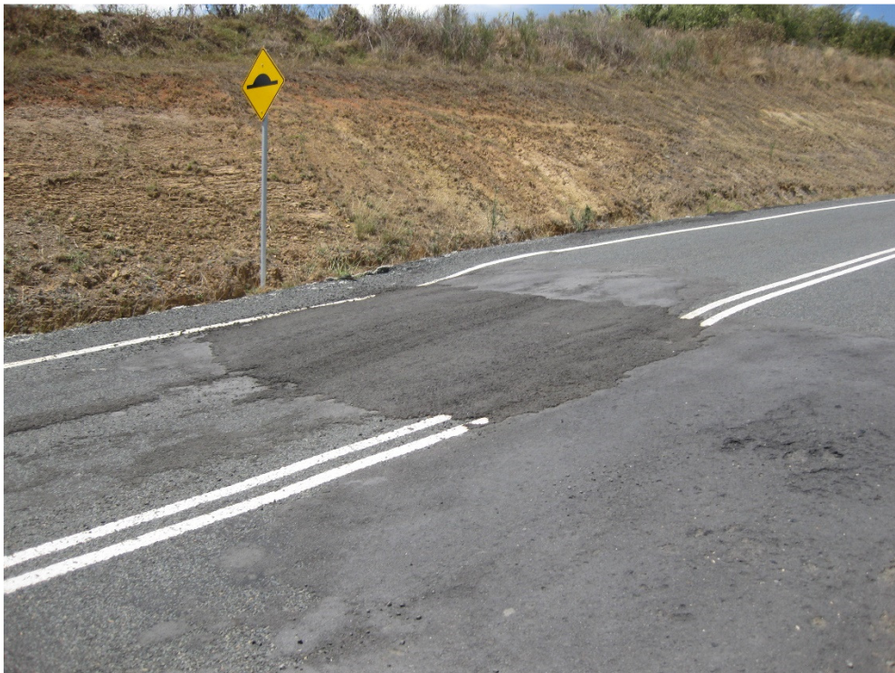
Photo 12 - Remediation works to Public Road impacted by Subsidence above Area 7
