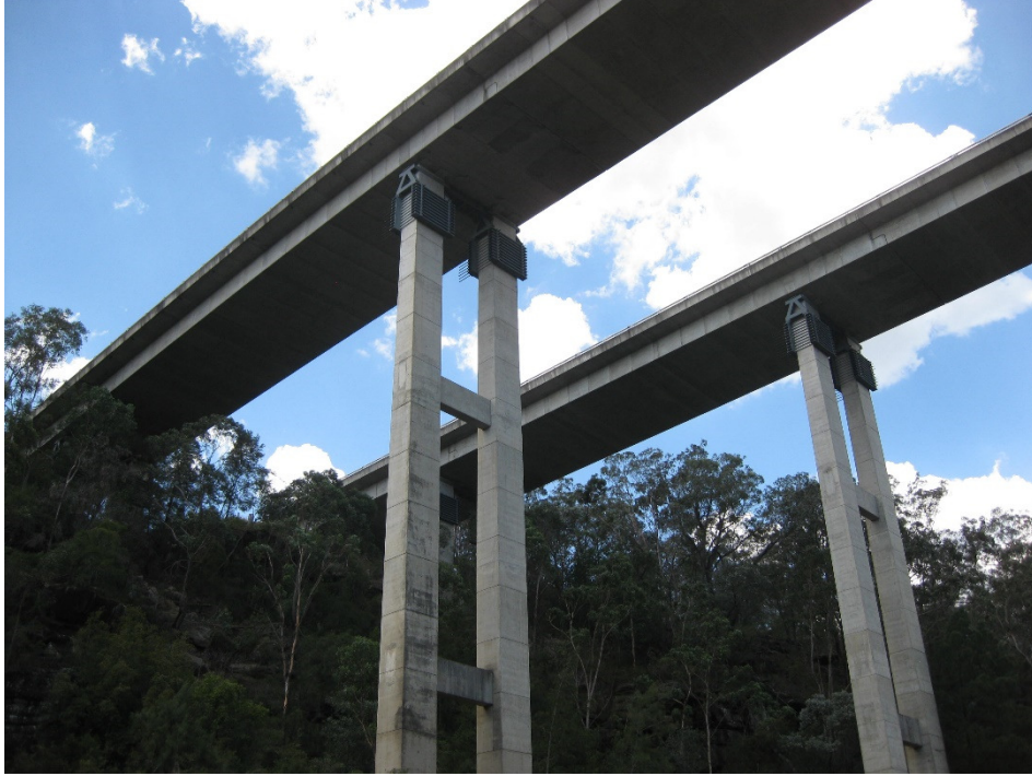
Photo 9 - Hume Highway Twin Bridges above Nepean River Crossing with Relevelling Gantry for Subsidence Remediation if Required
