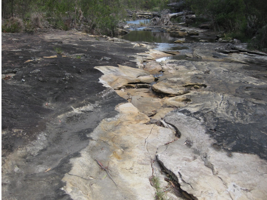
Photo 3 - Cracking Impacts to Georges River Rock Bar adjacent to LW35 - Level 2 Impact (sub-surface flow diversion that re-surfaces down stream)
