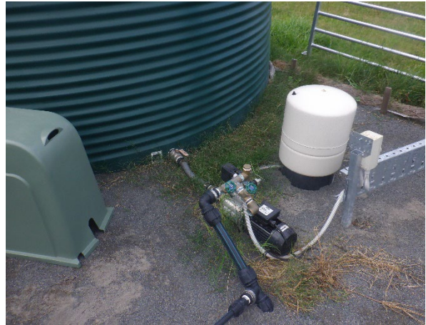
Photo 4: Borehole GW101986 and pump. Taken on 20/04/2023.
