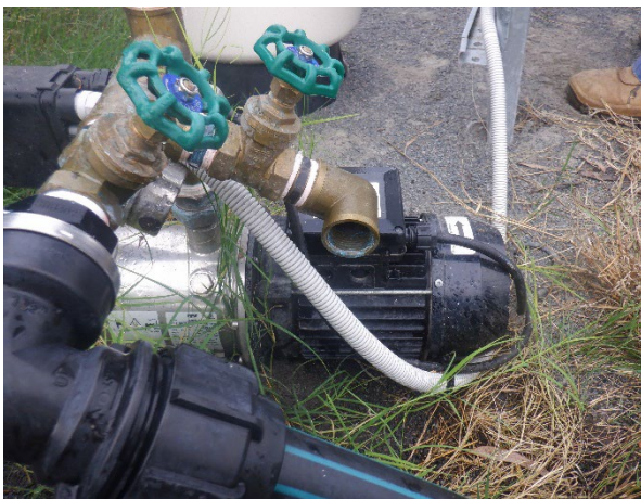
Photo 5: Borehole GW101986 outflow and pump. Taken on 20/04/2023.
