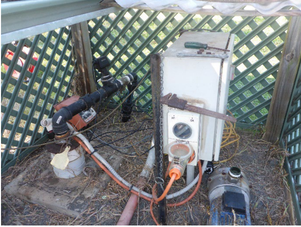
Photo 1: Borehole GW105534 and pump. Taken on 23 August 2017.
