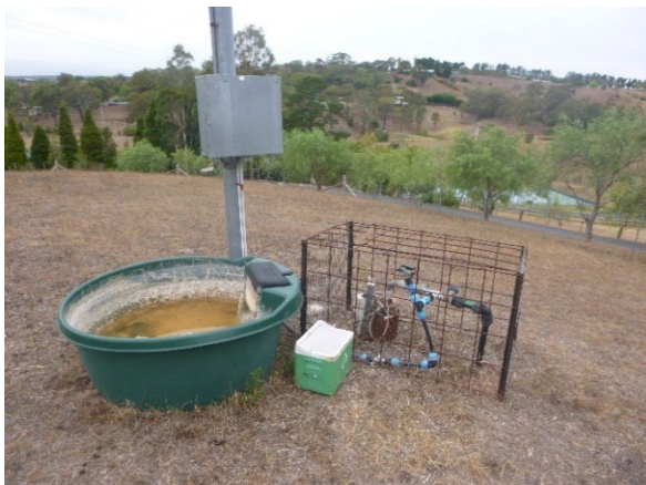
Photo 1: Photo of GW101986 and pump. Taken on 22/2/2018.
