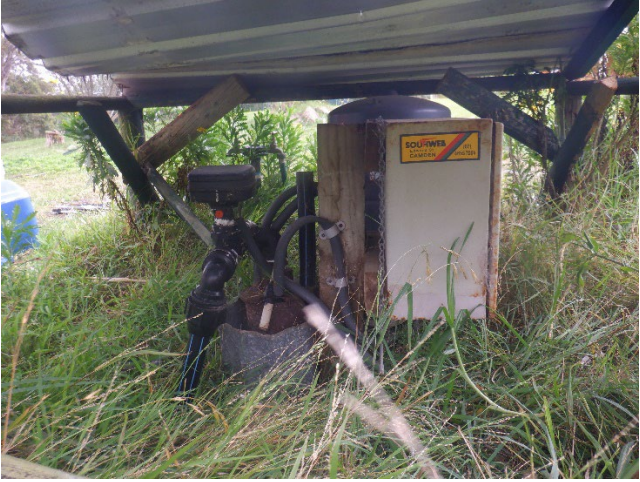
Photo 12: Borehole GW072249 – pumping equipment. Taken 20 April 2023.
