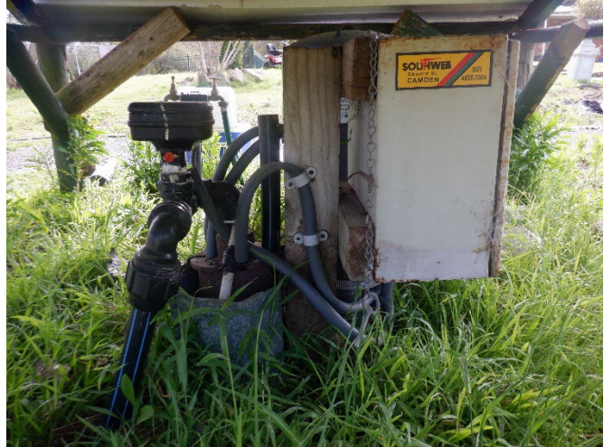
Photo 8: Borehole GW072249 – pumping equipment. Taken on 26 August 2022.
