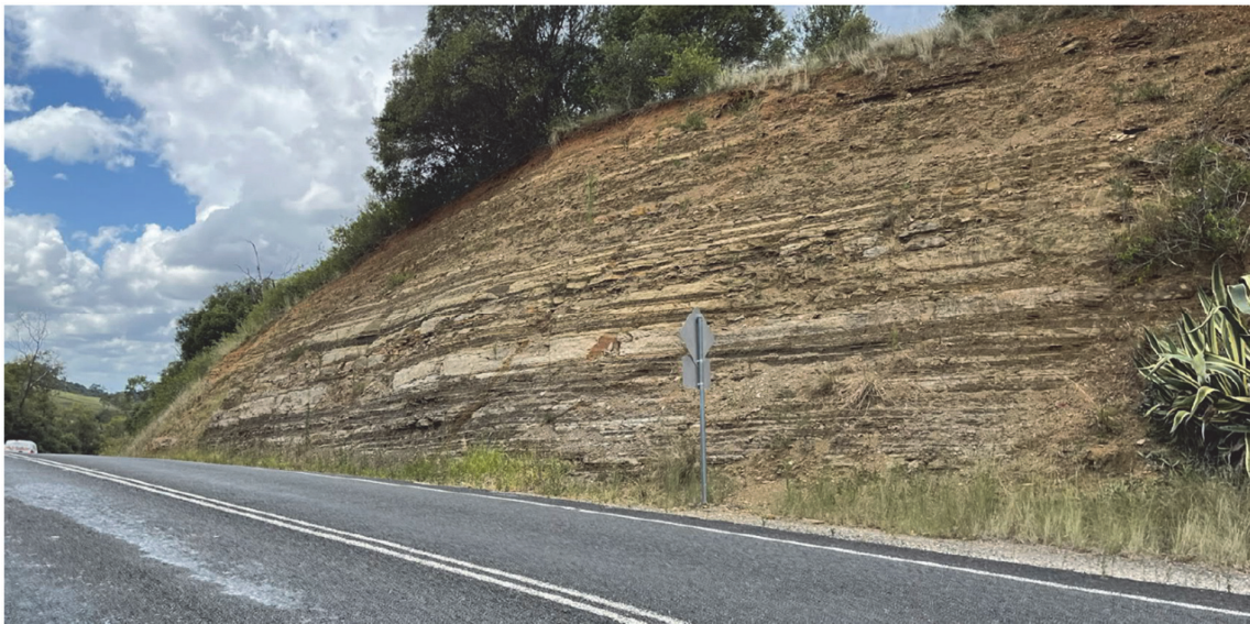
Fig. 3.3 Minor fretting and dislodgment of small rocks in rock cutting between MR9083 and MR9088 (Source: SLR, photograph taken on 2 March 2023)
