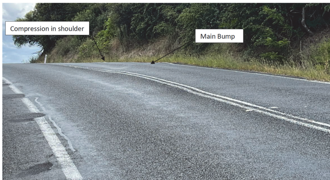
Fig. 3.1 Bump in eastbound lane and compression in shoulder along Menangle Road between Marks MR9085 and MR9086 (Source: SLR, photograph taken on 2 March 2023)
