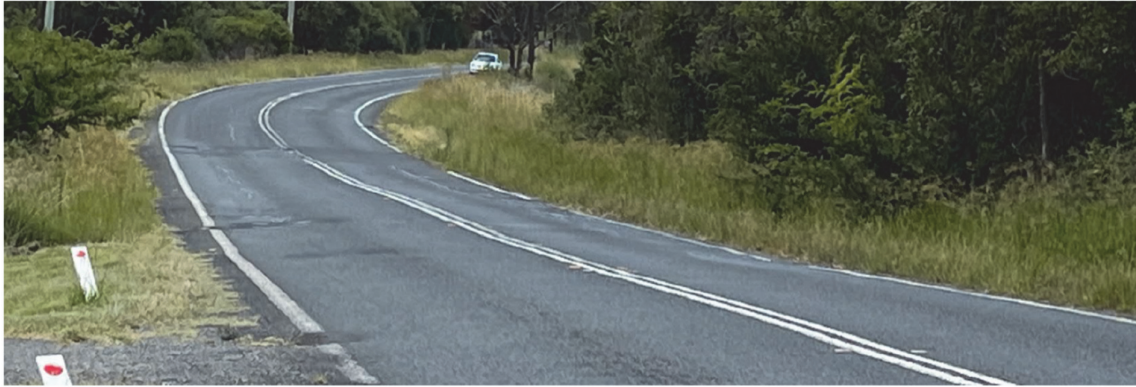
Fig. 3.2 Deterioration of pavement between MR9097 and MR9098 likely due to heavy rainfall and traffic load (Source: SLR, photograph taken on 2 March 2023)
