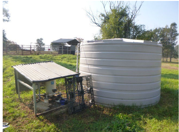
Photo 6: Settling tank where water from GW100673 is pumped. Photo taken on 29 April 2021.
