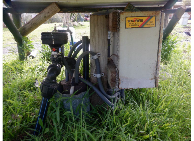
Photo 8: Borehole GW072249 – pumping equipment. Taken on 26 August 2022.
