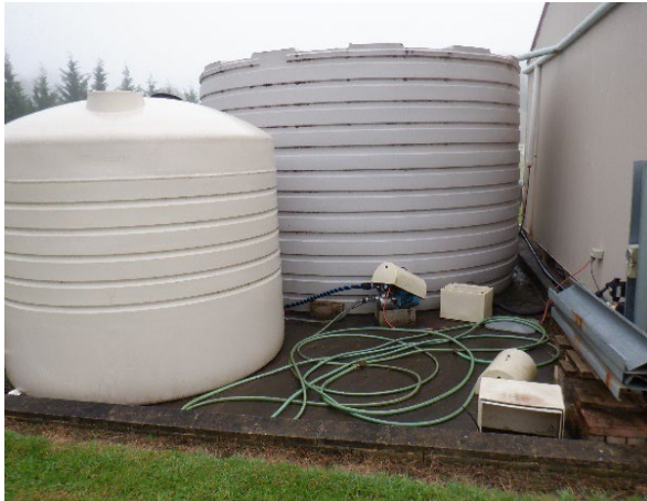
Photo 7: Electric pump for GW110671, photo taken on 25 May 2021.
