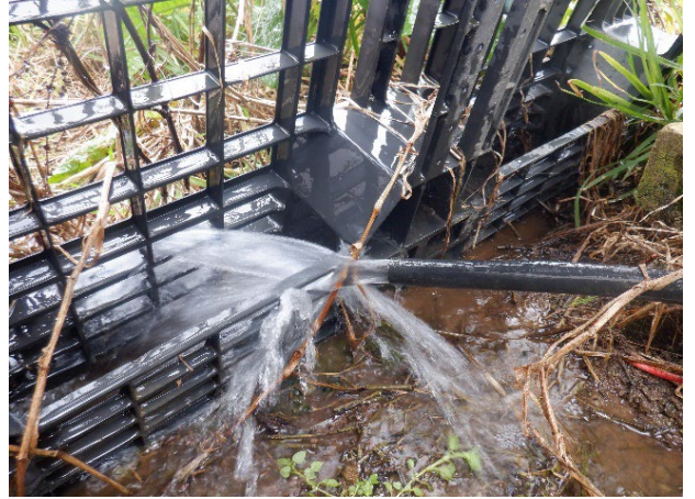
Photo 8: Discharge coming out of a hose with a valve from borehole pump. Photo taken on 26 August 2022.
