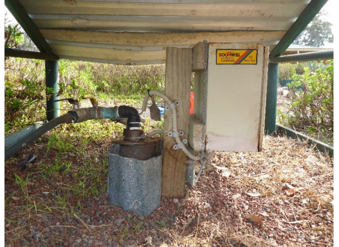
Photo 2: Borehole GW072249 – pumping equipment. Taken on 2 November 2017.
