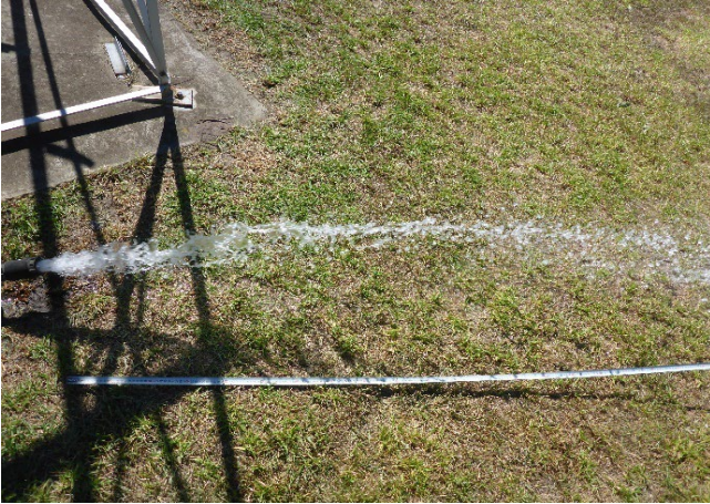
Photo 1: Water pressure from pump. Taken on 16 April 2018.
