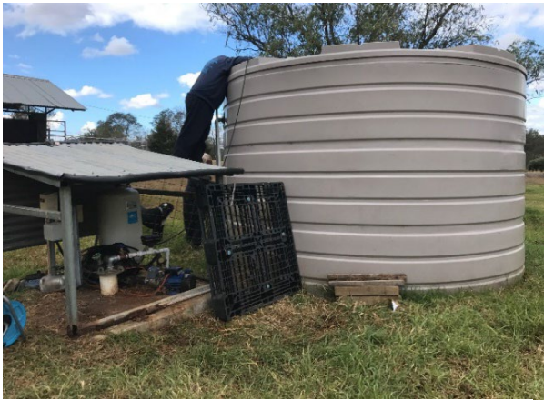
Photo 3: Settling tank where water from GW100673 is pumped. Photo taken on 16 May 2018.
