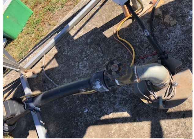
Photo 2: Closeup of borehole GW104602. Taken on 16 April 2018.
