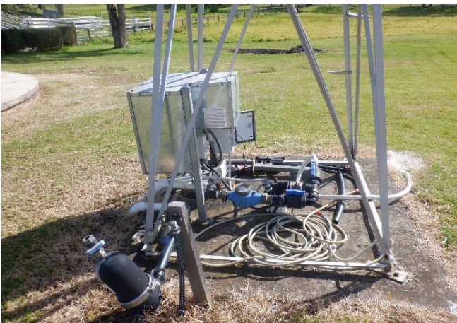
Photo 9: Borehole GW104602 showing the current set-up. Taken on 26 August 2022.
