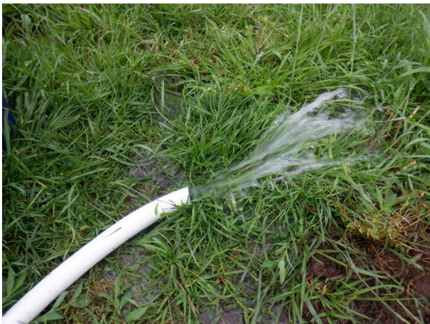
Photo 17: Discharge coming from hose on borehole. Taken 5 October 2022.
