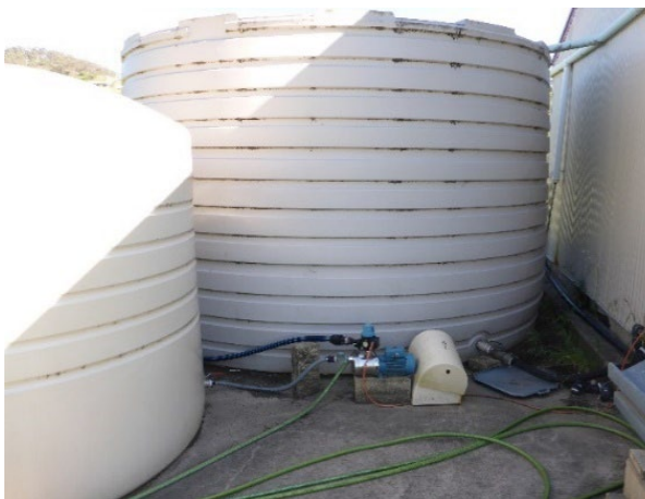
Photo 3: Electric pump for GW110671, photo taken on 15 November 2017.
