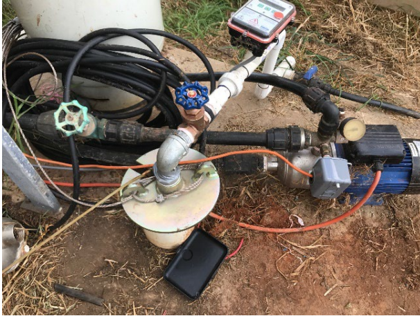
Photo 1: The capped borehole GW100673. Photo taken on 16 May 2018.
