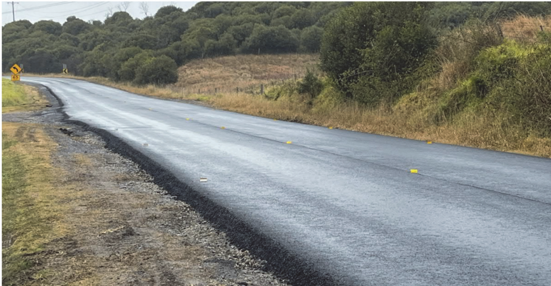
Fig. 3.2 Slight bump in pavement along Menangle Road between Marks MR9068 and MR9069 after completion of resurfacing works (Source: SLR, photograph taken on 20 July 2022)
