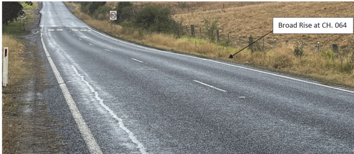
Fig. 3.1 Broad rise in pavement along Menangle Road between Marks MR9064 and MR9065 (Source: SLR, photograph taken on 20 July 2022)
