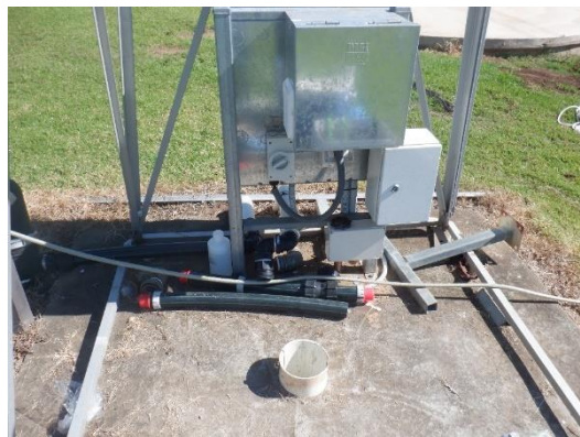
Photo 7: Borehole GW104602 showing the current set-up and pump removed. Taken on 3/5/2021.
