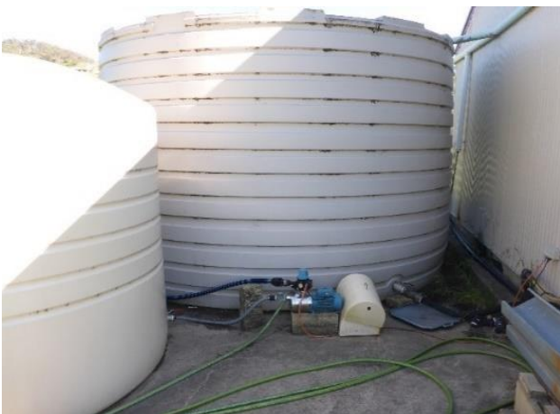
Photo 3: Electric pump for GW110671, photo taken on 15 November 2017.
