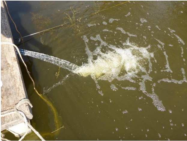
Photo 1: Borehole outlet into Dam 1. Taken on 2 November 2017.
