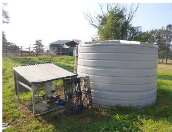
Photo 6: Settling tank where water from GW100673 is pumped. Taken 29 April 2021.
