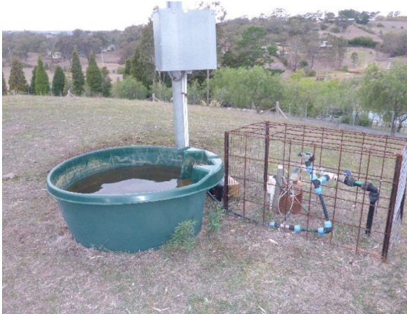
Photo 3: Borehole GW101986 and pump. Taken on 6/08/2018.
