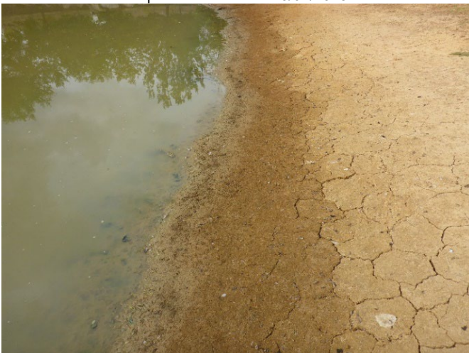
Photo 5: Soil cracking present around extent of dam edges observed during pre-mining inspection. Taken on 19/02/2018.
