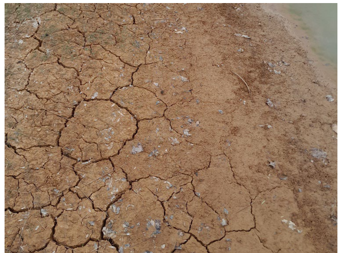
Photo 6: Soil cracking present around dam edges. Taken on 28/09/2023
