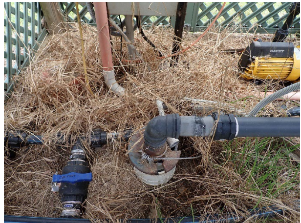
Photo 2: Borehole GW105534 and pump. Taken on 28 September 2023.
