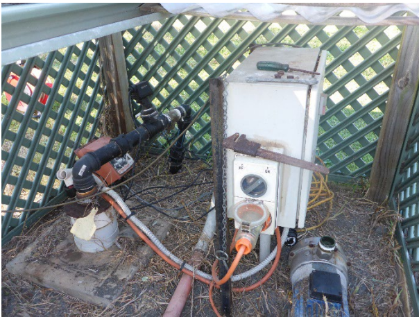
Photo 1: Borehole GW105534 and pump. Taken on 23 August 2017.
