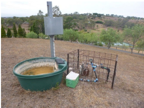
Photo 1: Photo of GW101986 and pump. Taken on 22/2/2018.
