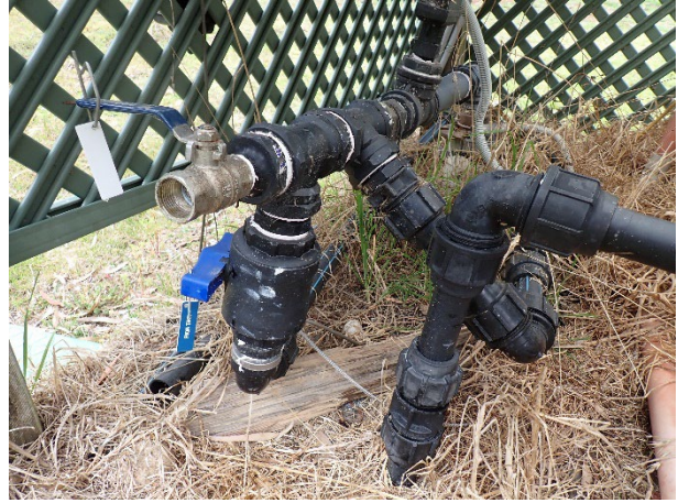
Photo 6: GW105534 outlet discharge. Taken on 28 September 2023.
