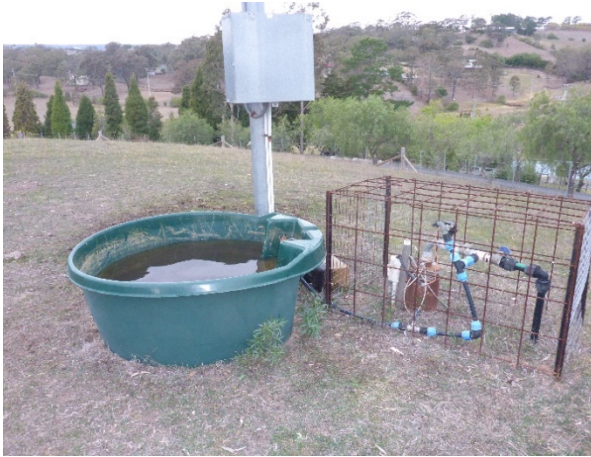
Photo 3: Borehole GW101986 and pump. Taken on 6/08/2018.
