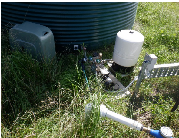
Photo 5: Borehole GW101986 and pump. Taken on 17/03/2022.
