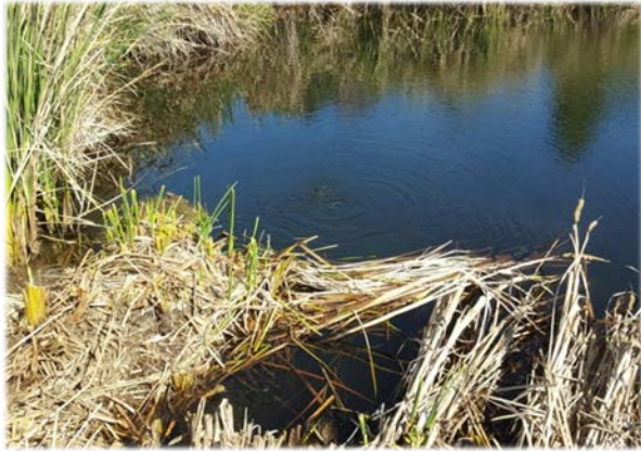
Photo 1: E13d01, gas bubbling from dam. Taken 6th April 2016.
