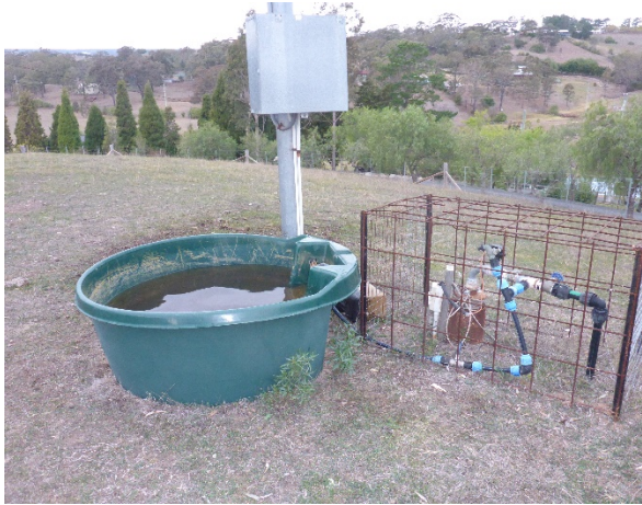
Photo 3: Photo of GW101986 and pump, taken 6/8/2018.
