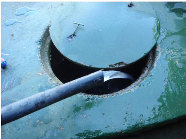
Photo 1: Flow from outlet pipe and storage tank during baseline inspection. Photo taken on the 11/10/13.
