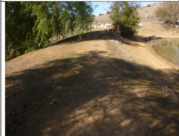
Photo 9: Image of dam wall during post-mining inspection, looking southeast. Taken on 25 th July 2018.
