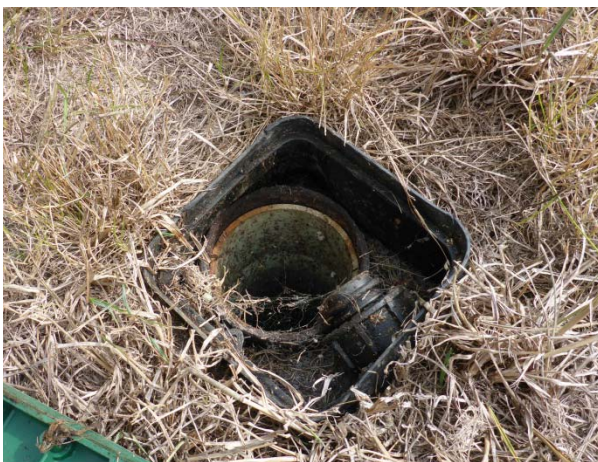
Photo 7: Picture of second borehole located on follow up inspection on 22/4/16. Photo taken on 22/4/16.
