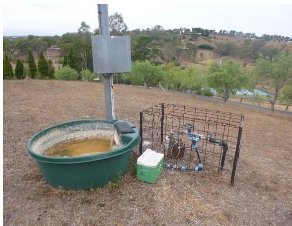
Photo 1: Photo of GW101986 and pump, taken 22/2/2018.
