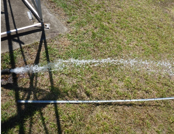
Photo 1: Water pressure from pump. Taken on 16/04/2018.
