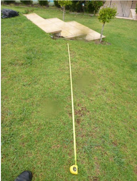
Photo 1: Longest identifiable soil crack on landholder's property. Taken on 04/01/2016.
