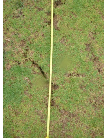
Photo 5: AA7_LW706_003; widest identifiable crack on landholder's property. Taken on 04/01/2016.
