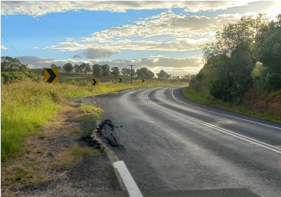
Figure 4.1 Pavement Heaving and Bleeding
