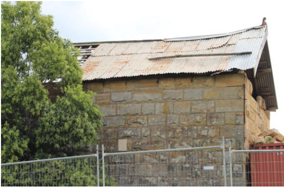
Plate 11. Closer view of remaining roof on western side of the building.
