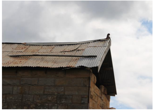
Plate 12. Closer view of remaining roof on western side of the building.
