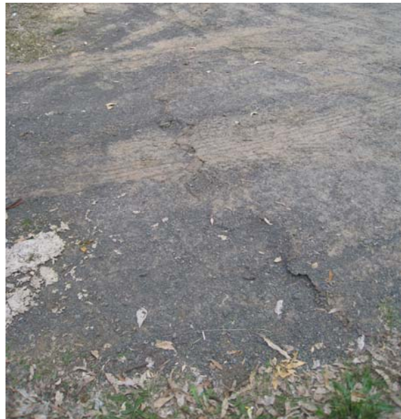
Fig. 4.12 Surface Compression Buckling Observed in a Pavement
