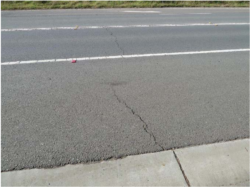
Fig. 6.1 Transverse Cracking (Photograph Courtesy of Colin Dove)
