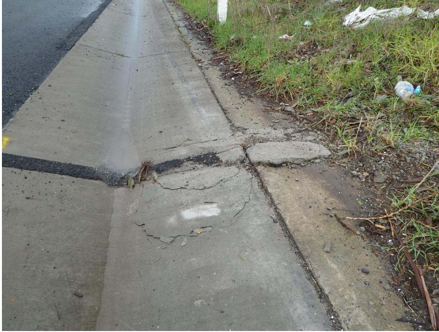
Fig. 6.3 Spalling of concrete kerb (Photograph Courtesy of Colin Dove)
