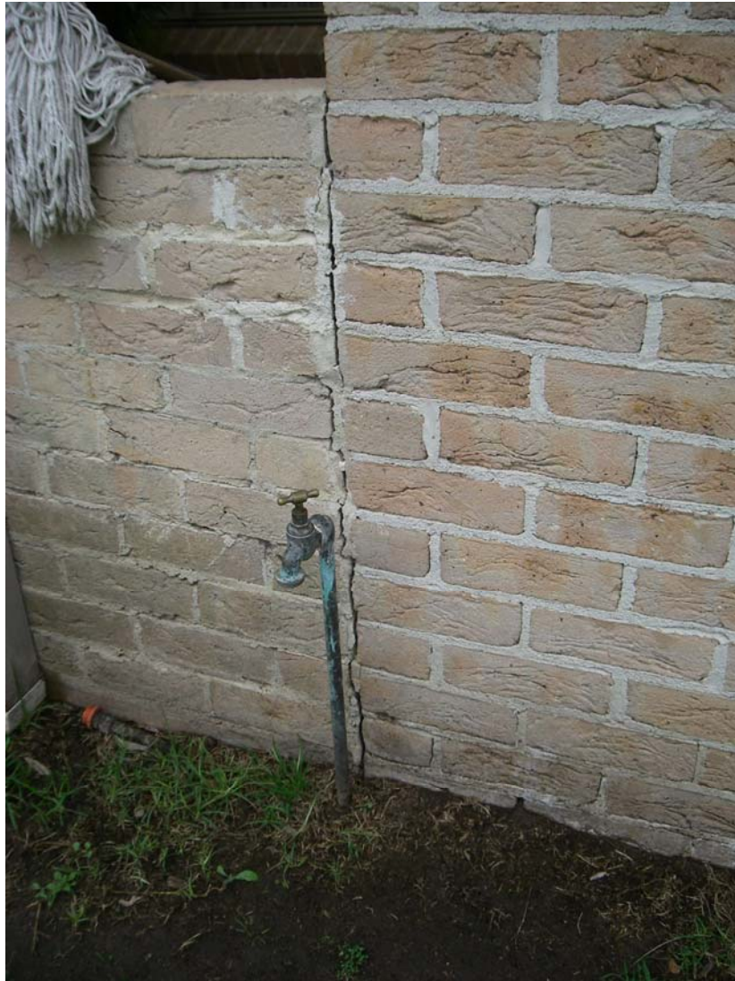
Fig. C.2 Example of crack in mortar only
