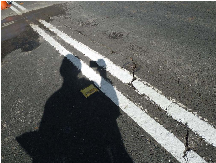
Fig. 6.4 Shear cracking (Photograph Courtesy of Colin Dove)
