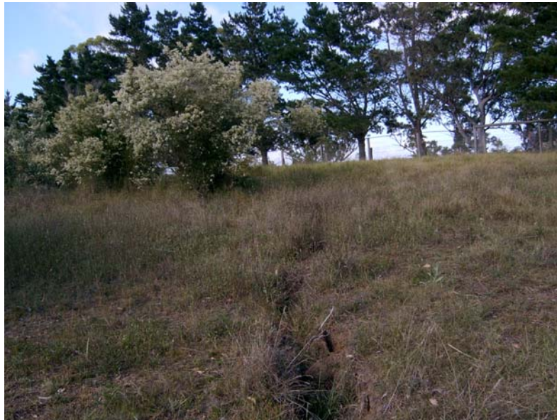
Fig. 5.16 Example of Surface Tension Cracking along the Top of a Steep Slope
