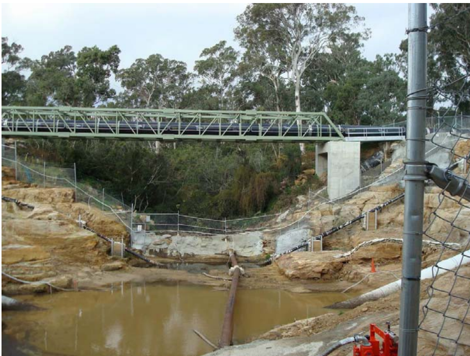
Plate 4.b. Extensive earthworks within the channel of Mallaty Creek associated with the Eastern Gas pipeline.
