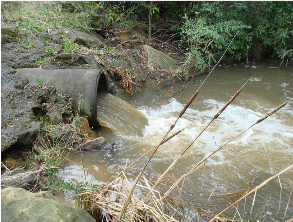
Plate 4 a. Pipe culvert at Blackburn Road crossing of Georges River creating a barrier to fish passage.
