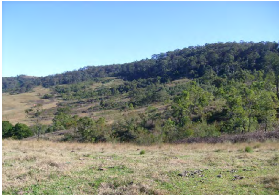
View to Southwest Looking Across Numerous Landslides on Slopes Below Tree Covered Escarpment
