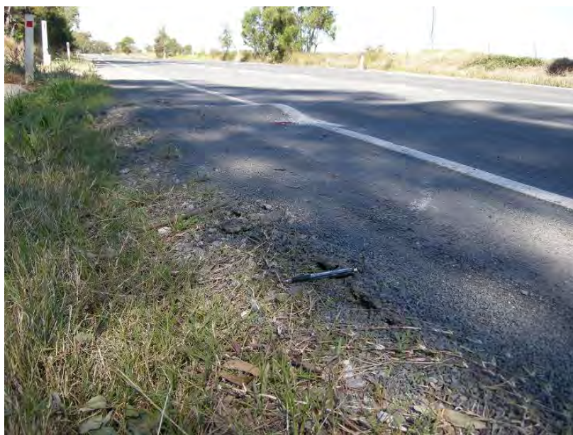
Fig. 6.28 Bump in Slip Lane along Appin Road above West Cliff Longwall 32 (Courtesy of Colin Dove)
