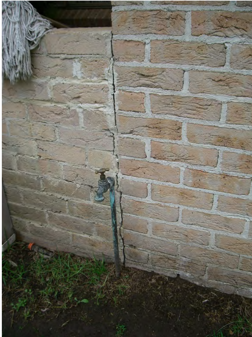
Fig. C.2 Example of crack in mortar only
