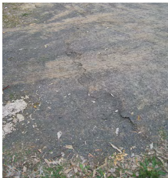
Fig. 4.12 Surface Compression Buckling Observed in a Pavement
