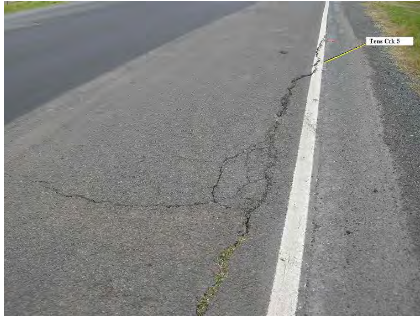
Fig. 6.29 Tension Crack in Appin Road above West Cliff Longwall 32 (Courtesy of Colin Dove)
