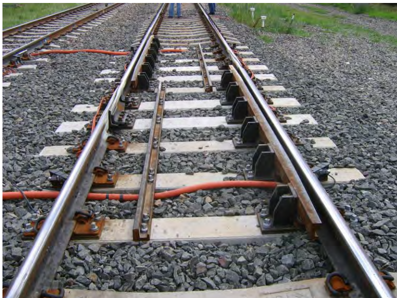
Fig. 6.3 Rail Expansion Switch
