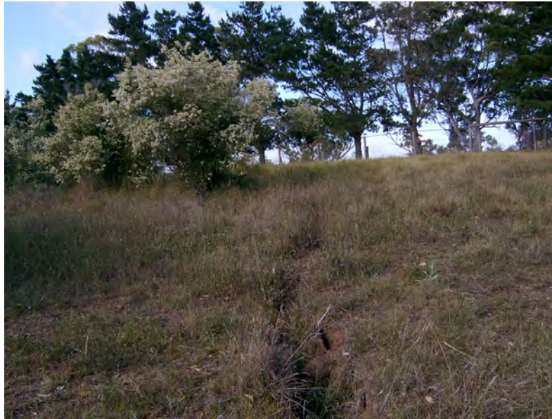
Fig. 5.31 Example of Surface Tension Cracking along the Top of a Steep Slope
