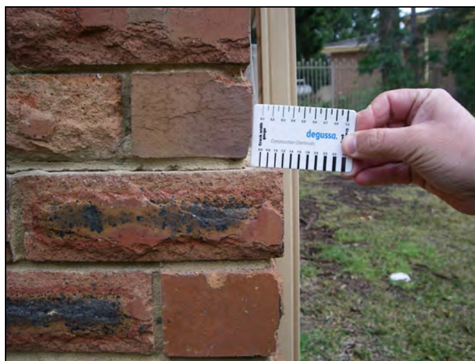
Fig. C.1 Example of slippage on damp proof course
