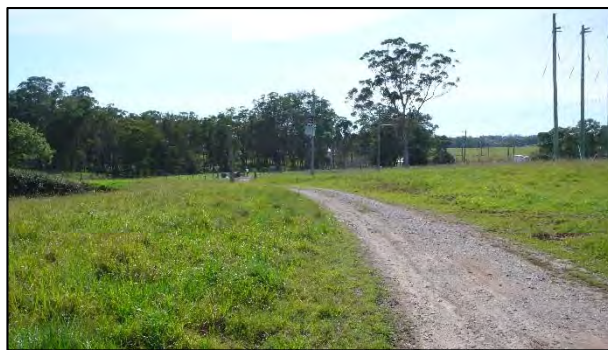
Plate 5: Example of low to moderate levels of disturbance through road construction and vegetation clearance.
