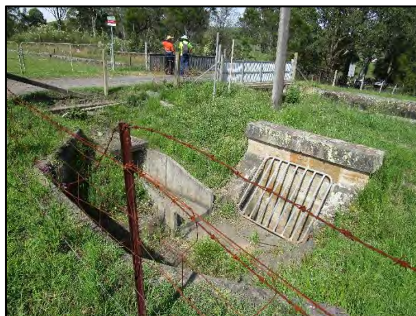
Plate 3: Sandstone culvert and discharge channel running beneath the Upper Canal on the north side of Brooks Point Road, looking south west.
