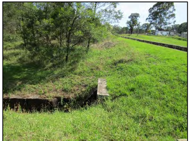
Plate 12: Sandstone discharge channel running west beneath the Upper Canal on the north side of Brooks Point Road, looking north.
