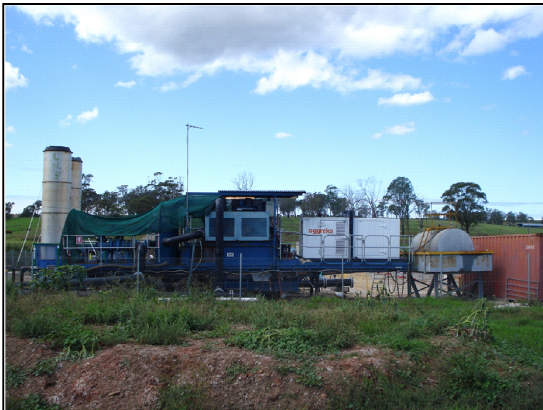
Figure 5.4 – Typical Trailer Mounted Gas Extraction Plant
