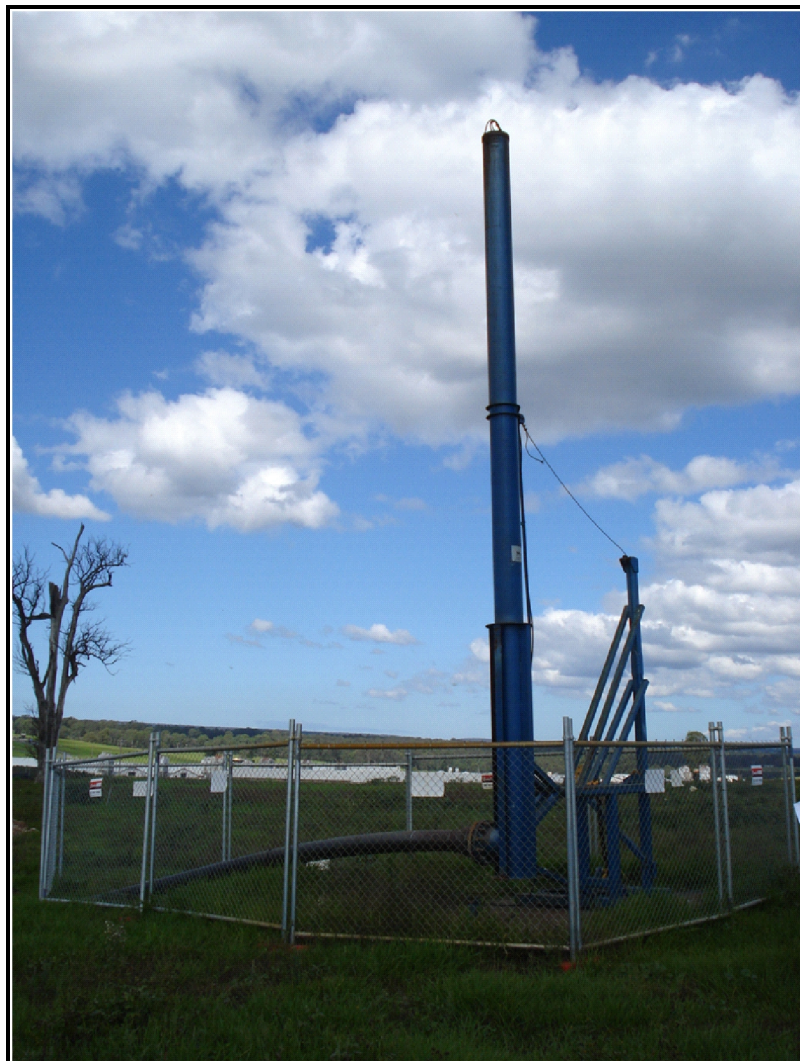
Figure 5.11 – Typical Vertical Gas Discharge Stack
