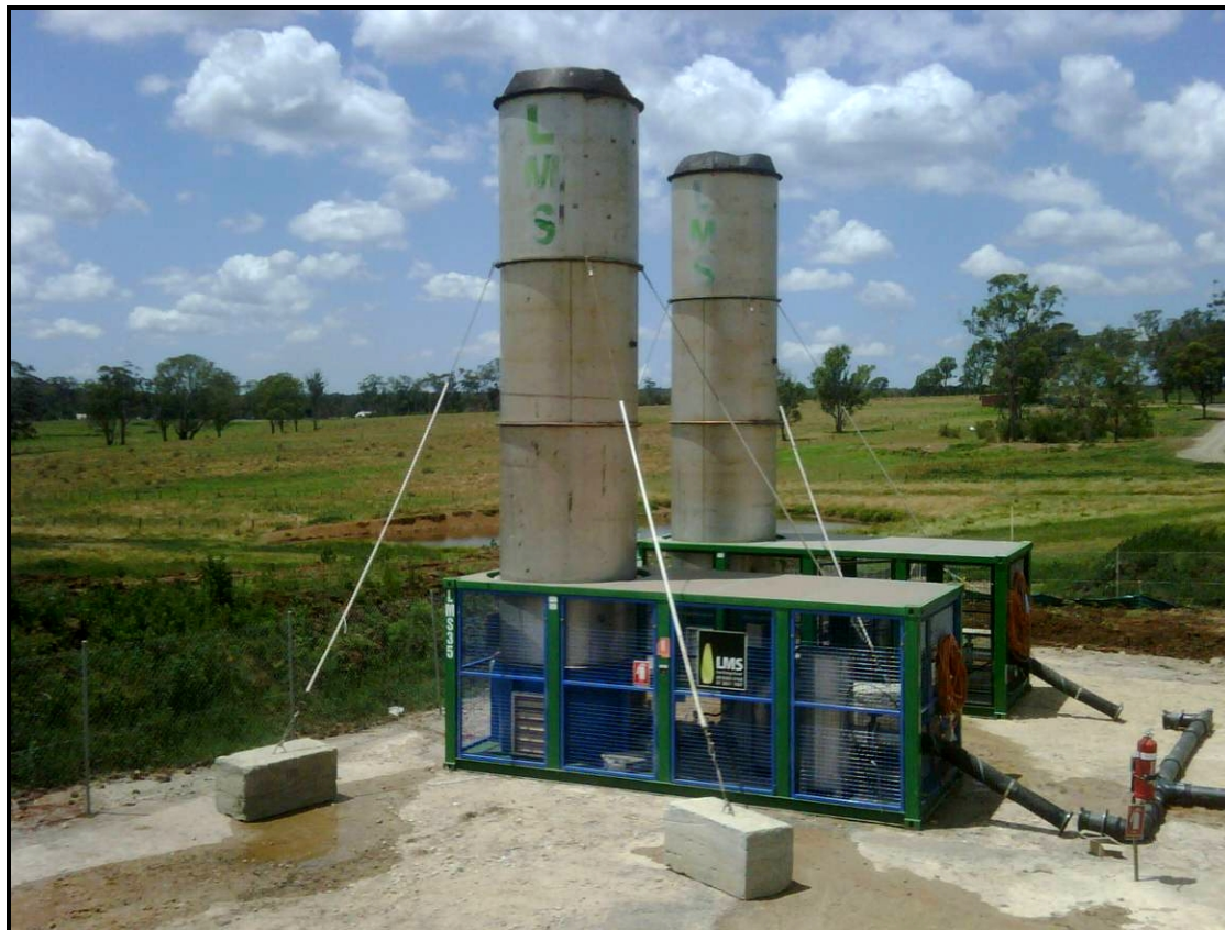
Figure 5.12 – Typical Enclosed Flaring Units
