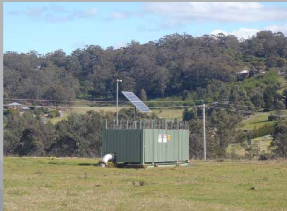
Once drilling activities are completed, the site is backfilled to restore original contour of the land and a small compound is constructed around the wellhead.
