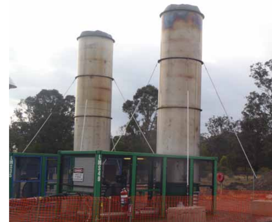
Where possible, gas from mine safety gas drainage holes is piped to methane gas power plants or in some cases is flared in enclosed flare stacks similar to those pictured above.
