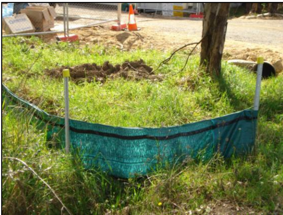
Figure 11 Sedimentation Control Structure
